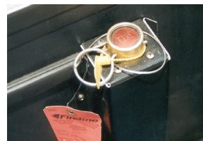
This system will put out the fire and prevent it from restarting.
