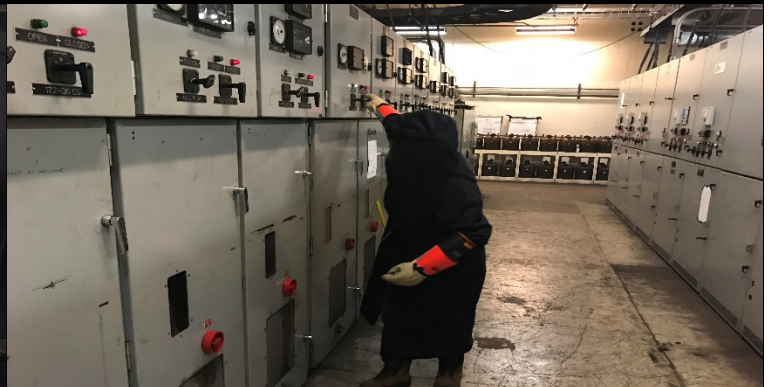
TRPM Technician Wearing FR 40 Cal Suit to Rack Breaker Back In
