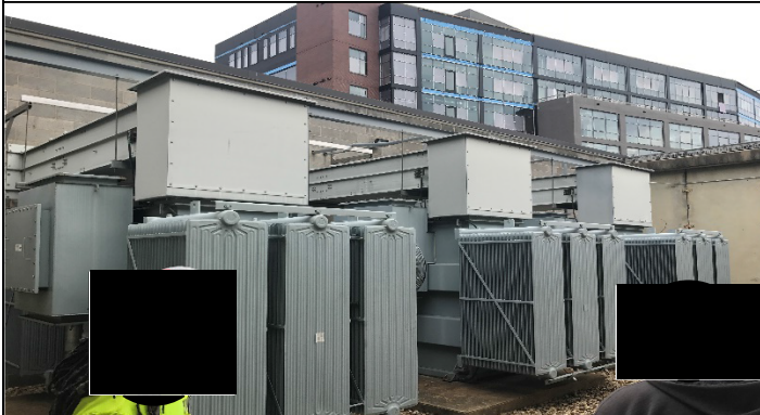
Transformers Outside TPSS Facility
