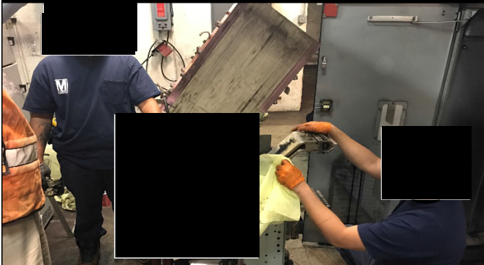
TRPM Technicians Cleaning Breaker
