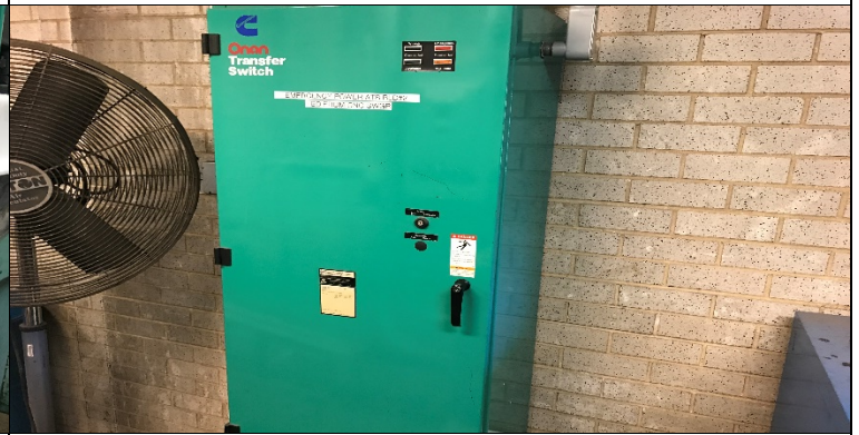
Generator Transfer Switch in Electrical Room
