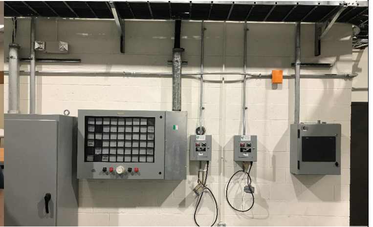
Figure 2: Annunciator Panel and DC Breaker Test Receptacles
