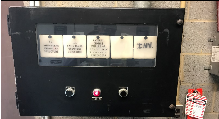
Annunciator Panel in AC Switchboard Room
