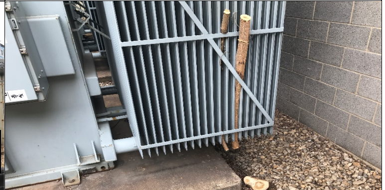
Tree branch Lodged in TPSS Transformer Radiator Fins
