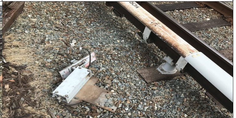
Destroyed Heater Tape Fuse Box near Control Panel
