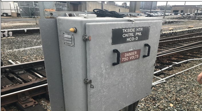
Trackside Heater Control Panel
