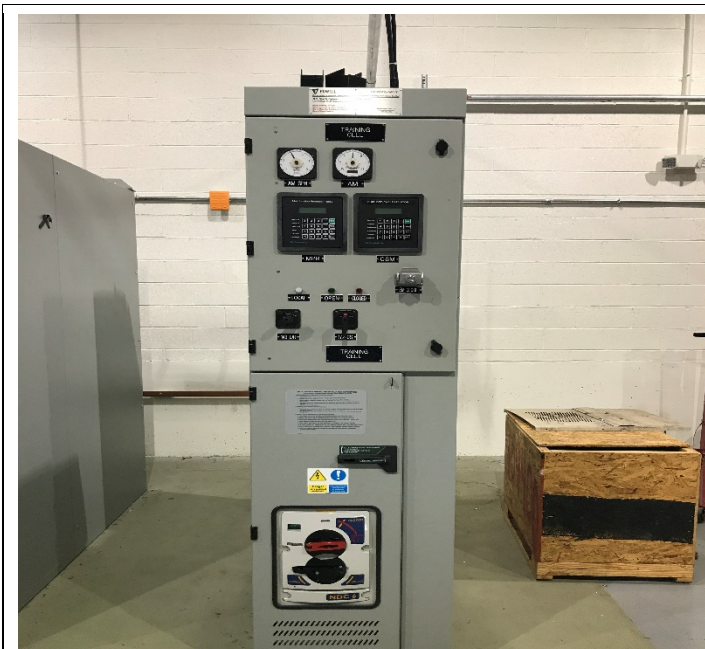
Figure 5: DC Breaker and new Smart Relays
