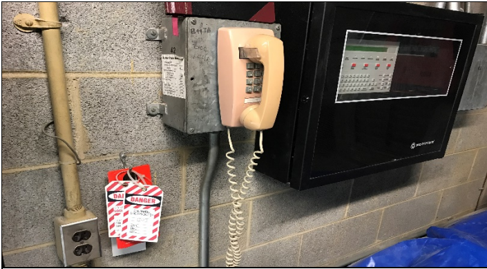
AC Switchboard Room Phone
