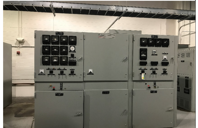
Figure 4: Auxiliary Panel with Metering and Control handles
