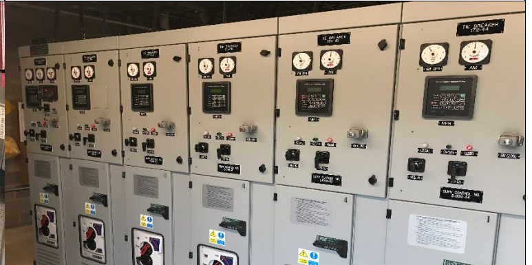
(B99) Brentwood Yard Tie Breaker Facility
