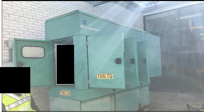
Diesel Powered Unit
