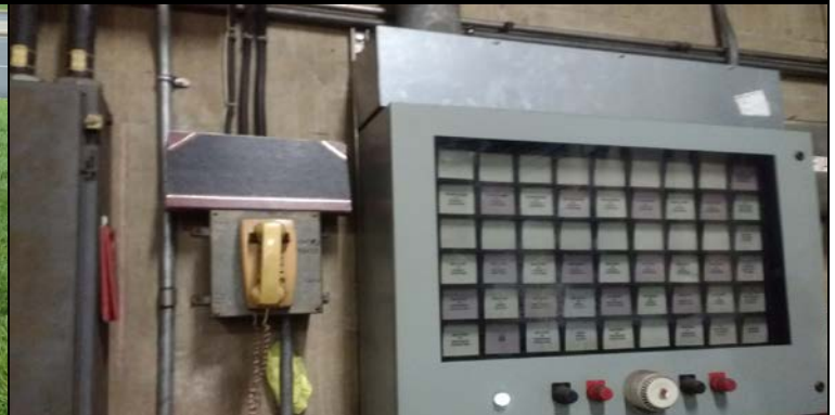
Figure 2: Annunciator Panel Showing No Issues
