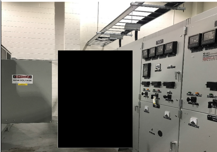
Figure 3: AC Switchgear Line Up
