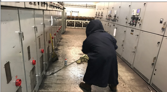
TRPM Technician Wearing FR 40 Cal Suit to Rack Out Breaker
