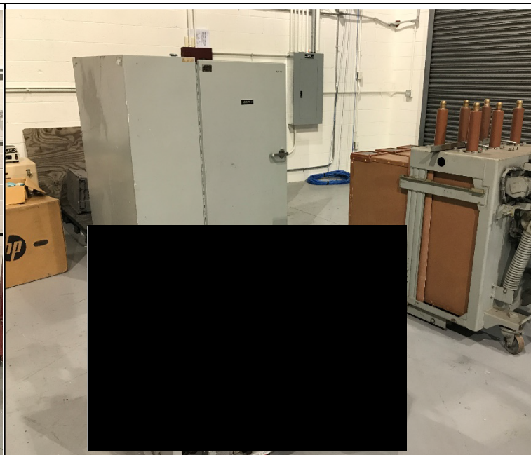
Figure 6: DC Breaker removed from cubicle for training
