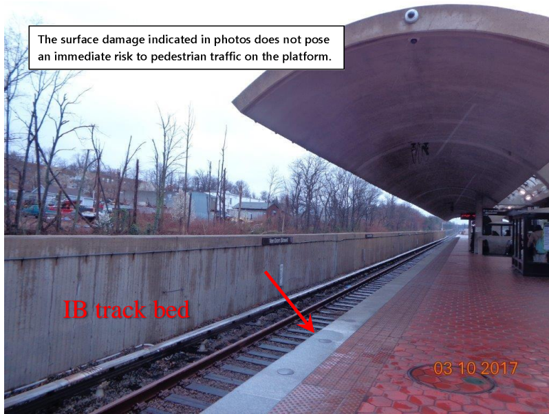
Figure 1: The location as marked is where the worst deterioration (approximately Chain Marker 690+00) is located.
