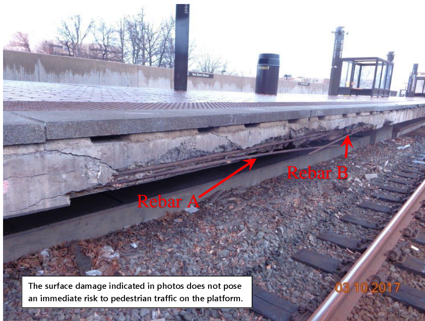
Figure 2: Side view of concrete deterioration and rebar corrosion/separation.
