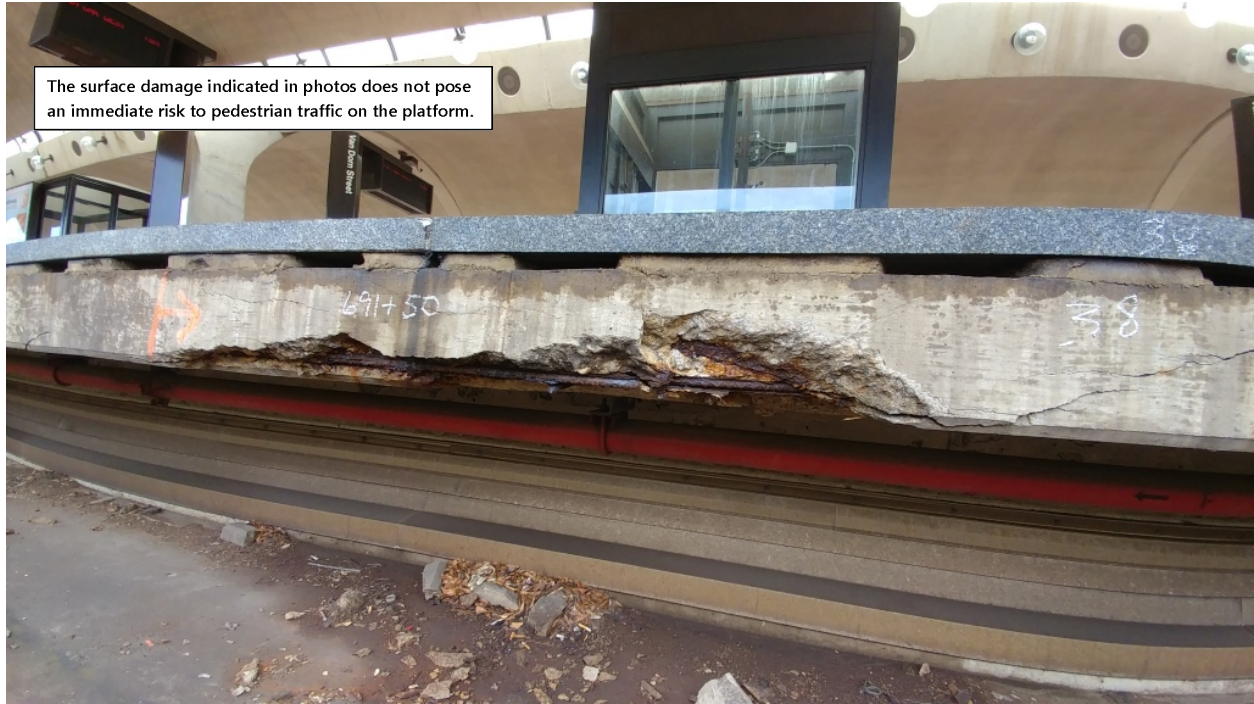
Figure 9: Large spall with exposed reinforcing steel at the edge of Track 2 platform, Chain Marker 691+50
