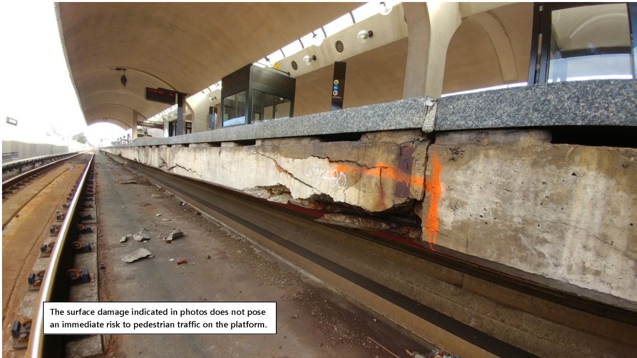
Figure 8: Large spall with exposed reinforcing steel at the edge of Track 2 platform, Chain Marker 691+80
