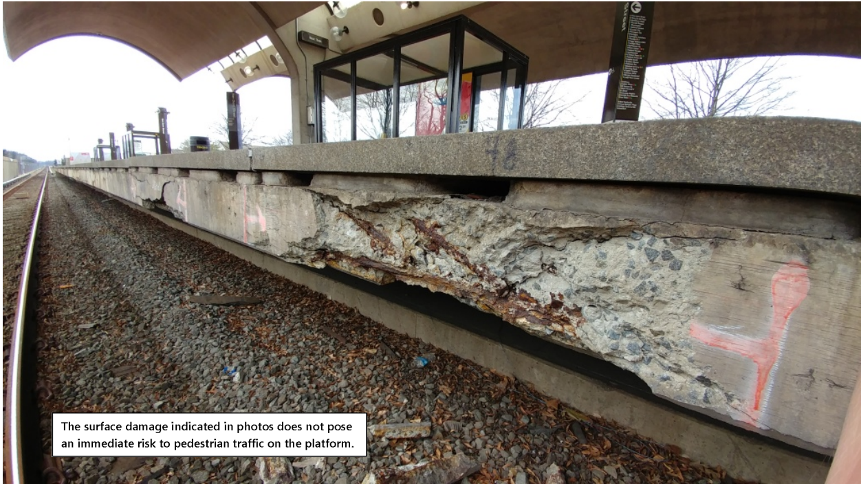
Figure7: Large spall with exposed reinforcing steel at the edge of Track 1 platform, Chain Marker 692+50
