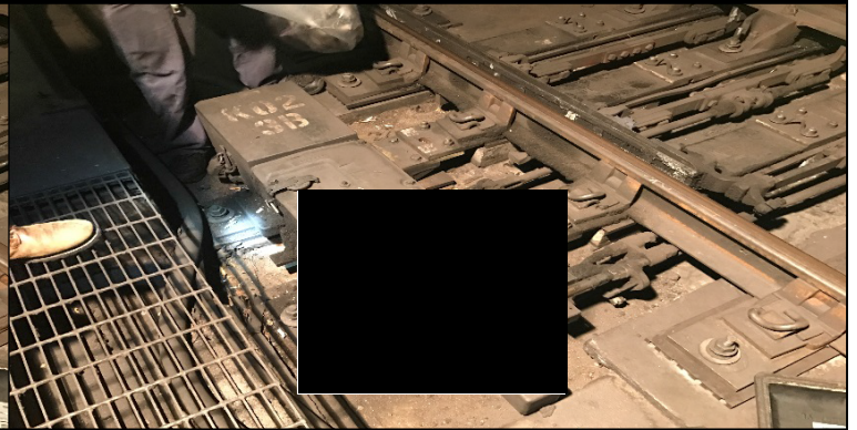
M3 Switch Machine with Cover Removed from Indication Box
