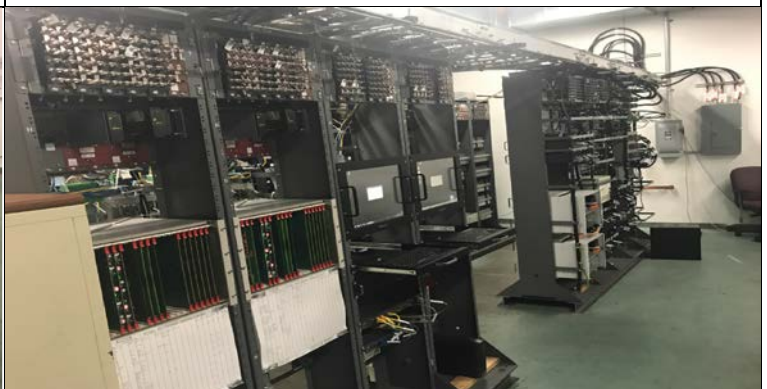
Figure 6: Programmable Logic Controllers (PLC) in ATC Lab #2
