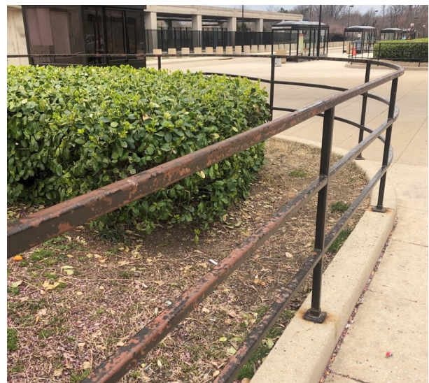
Pedestrian fencing, courtesy WMATA.
