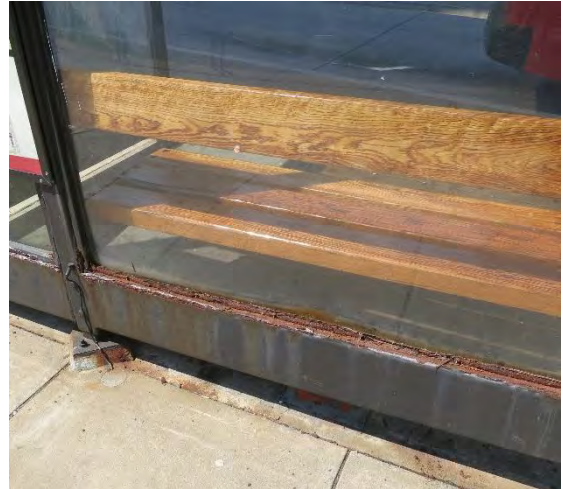
Figure 97: Frame Rust, Shelter D North
