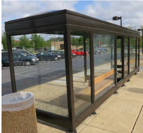
Figure 51: Missing Panel, Kiss & Ride
