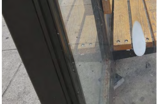
Figure 151: Frame Rust, Damaged Panel, Shelter M
