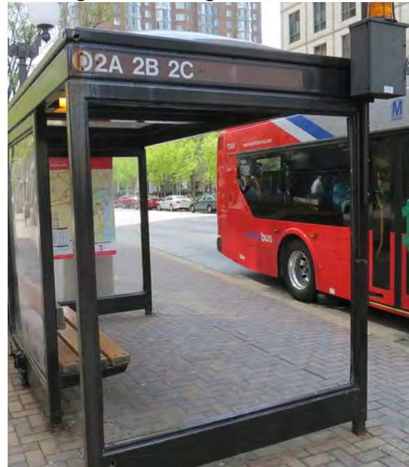
Figure 15: Missing Panel, Shelter D
