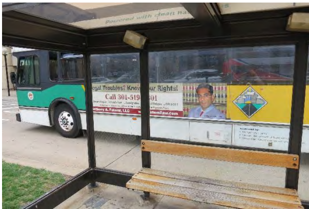
Figure 139: Kiss-and-Ride Shelter Missing Panel
