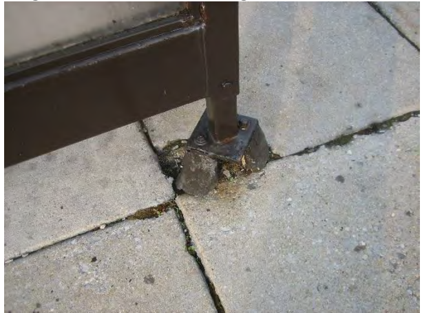
Figure 162: Cracked Footing and Pad, Shelter B
