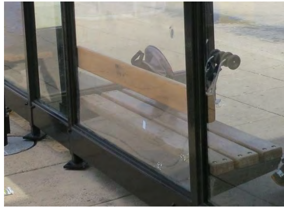
Figure 156: Worn Bench, Cracked Panel, Shelter L
