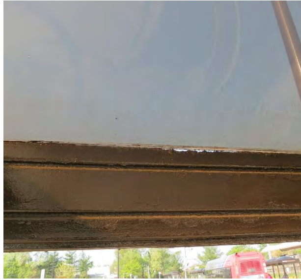
Figure 58: Frame Rust and Separated Dome Top, Kiss & Ride Shelter
