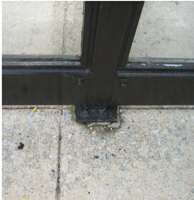
Figure 184: Cracked Pad & Footing, Shelter C
