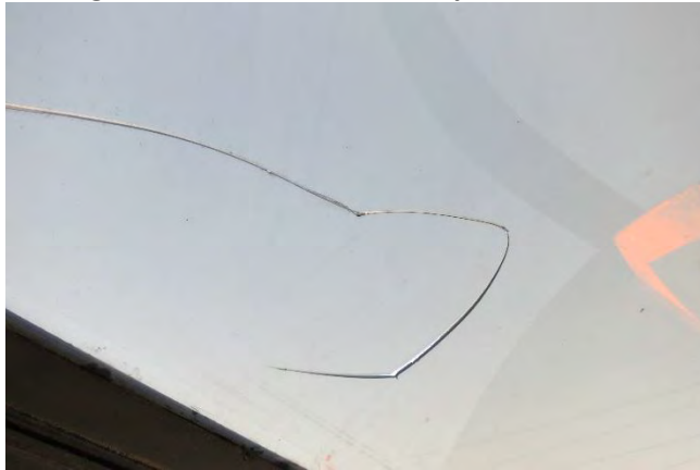
Figure 125: Cracked Dome Top, Taxi Shelter
