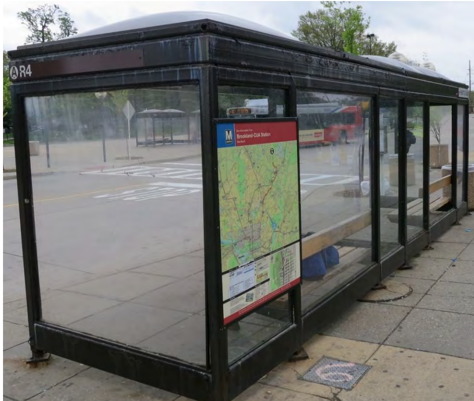
Figure 26: Poor Condition of Shelter A, Missing Panels, Missing Dome Top and Rust
