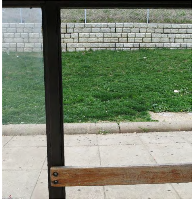
Figure 166: Shelter A East Missing Panel
