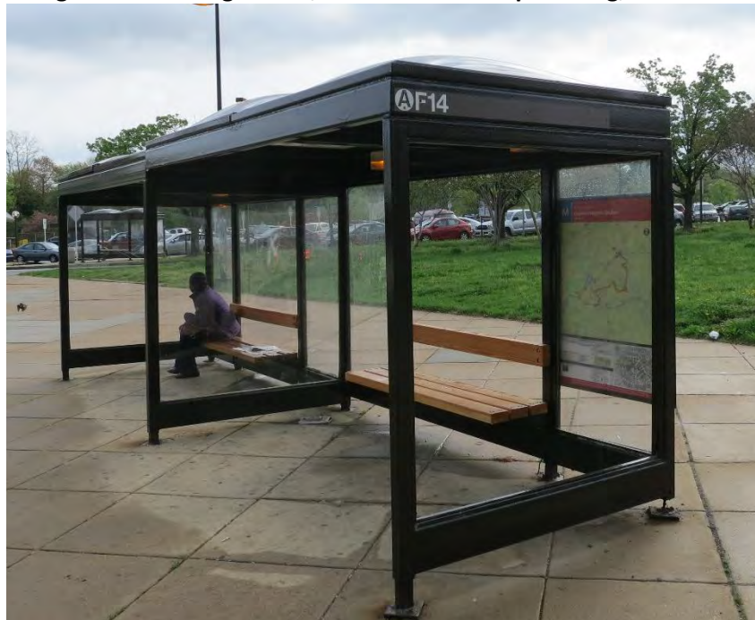
Figure 38: Missing Panels, Cracked Dome Top and Leg, Shelter A
