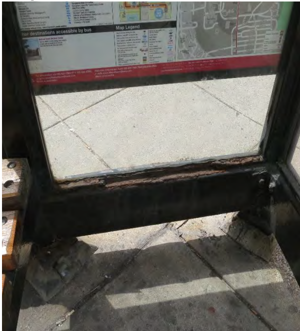
Figure 106: Poor Frame Condition, Shelter D
