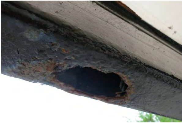
Figure 27: Hole in Frame, Shelter D/J
