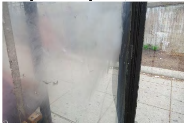
Figure 192: Damaged Panel, Shelter D
