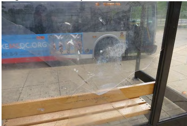
Figure 118: Severely Damaged Panel, Shelter F
