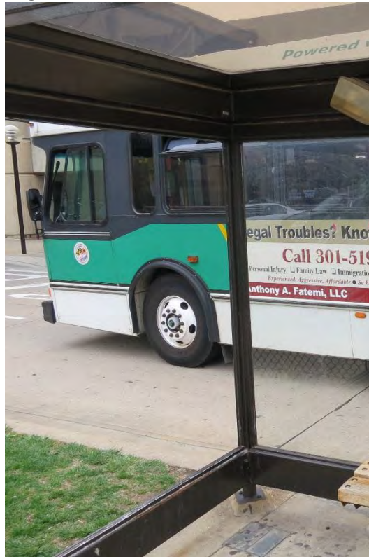
Figure 138: Shelter B West Rust on Frame
