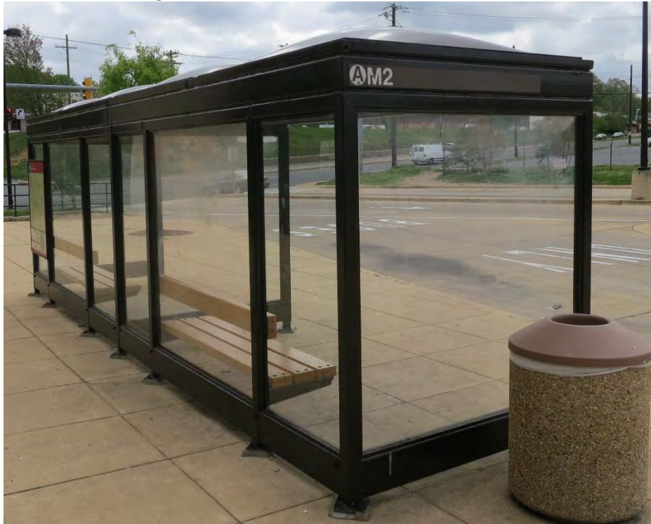
Figure 120: Good Frame Condition, Shelter A
