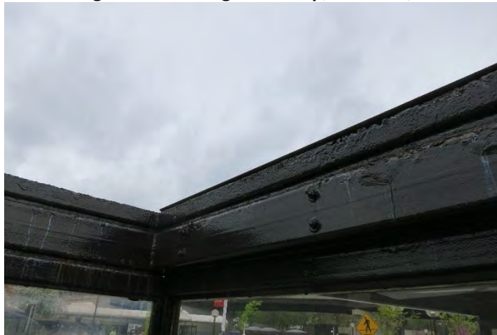
Figure 29: Missing Dome Top, Shelter E/H
