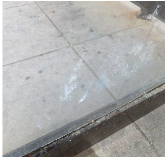
Figure 126: Panel Damage, Shelter A
