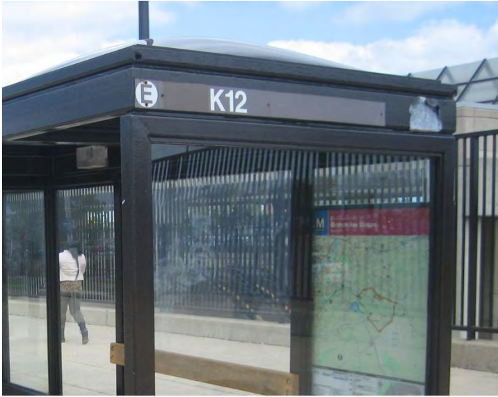
Figure 34: Peeling Paint, Shelter E
