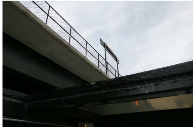
Figure 131: Missing Dome Top & Rust, Shelter C
