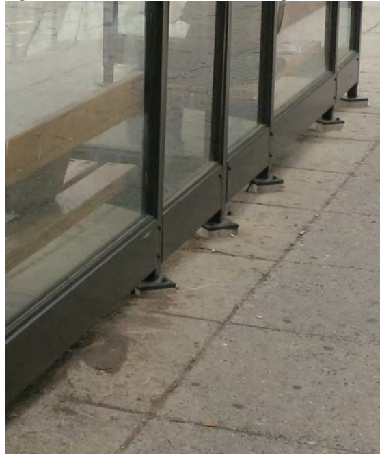
Figure 194: Cracked Pad & Footings, Shelter G
