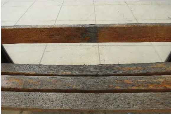
Figure 167: Shelter F East Poor Bench Condition
