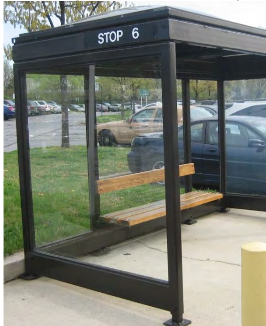
Figure 86: Missing Panel, Park-and-Ride Stop 6 Shelter
