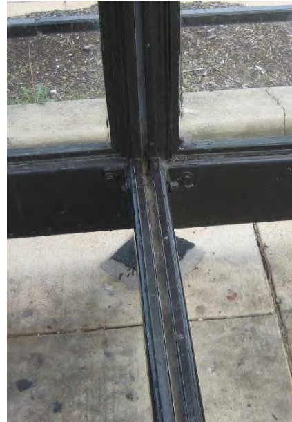
Figure 35: One of Two Missing Panels, East Kiss & Ride
