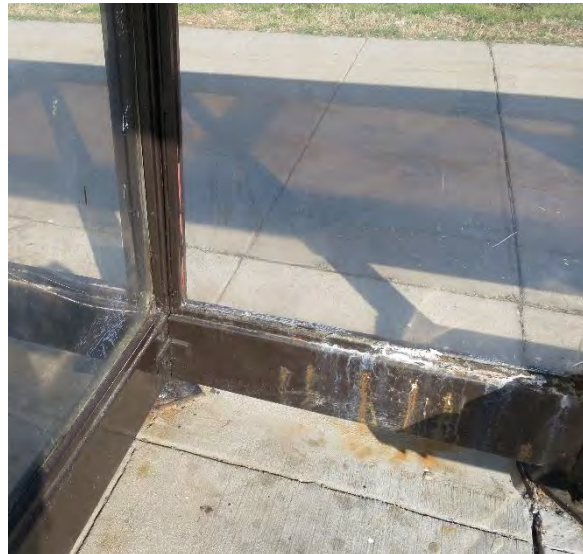
Figure 56: Frame Rust, Shelter C
