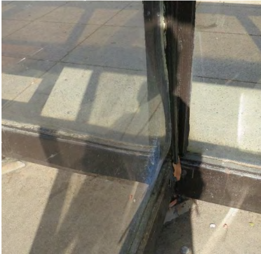
Figure 22: Damaged Panel, Shelter E
