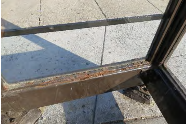
Figure 114: Frame Rust, Shelter B
