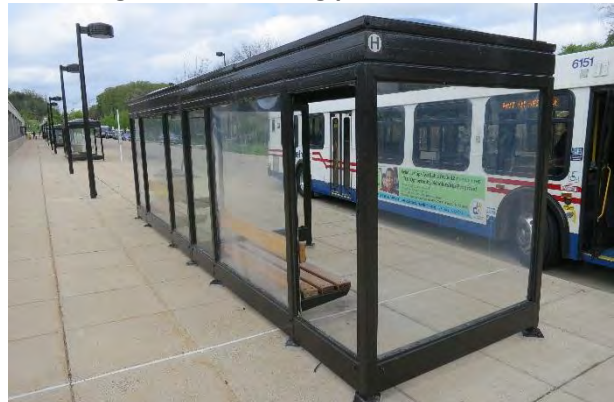
Figure 149: Missing panel, Shelter H
