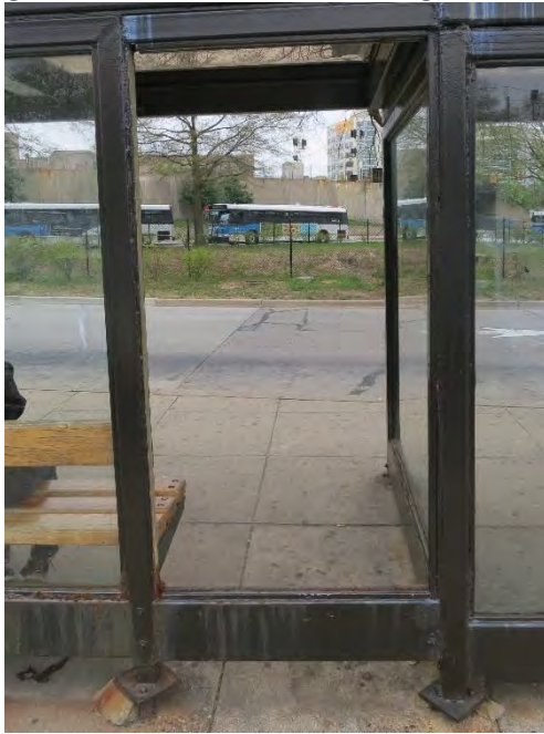
Figure 137: Shelter C East Missing Panel
