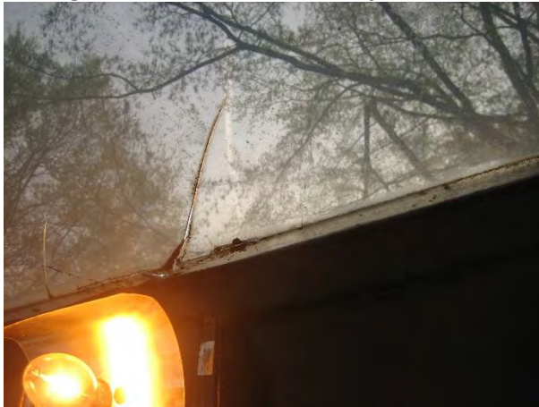
Figure 161: Cracked Dome Top, Shelter G
