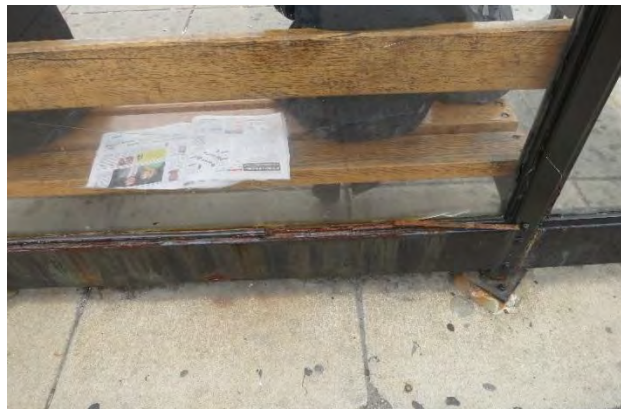
Figure 140: Shelter C East Poor Pad Condition
