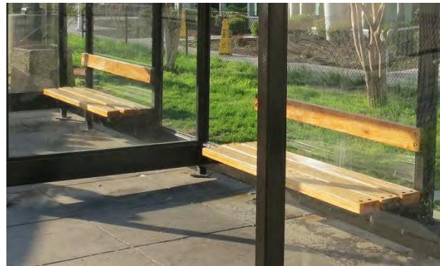
Figure 113: Worn Benches, Shelter G
