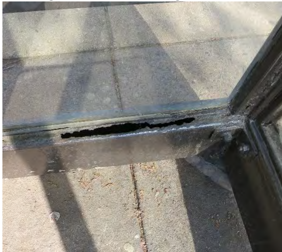
Figure 20: Frame Damage, Shelter B
