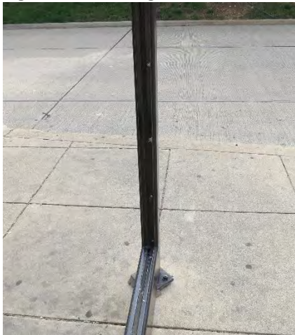
Figure 49: Missing Panel, Shelter D
