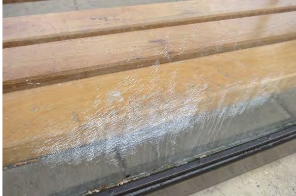
Figure 150: Damaged Panel, Shelter C
