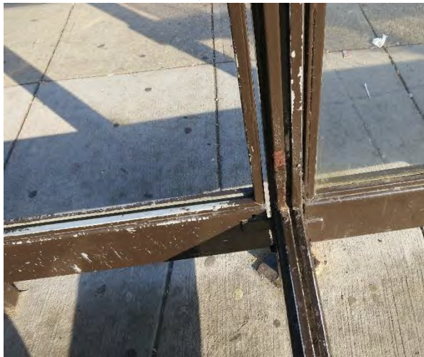
Figure 112: Missing Panel, Scratched/Rusted Frame, Shelter C
