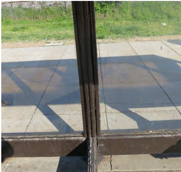
Figure 55: Missing Panel, Shelter B
