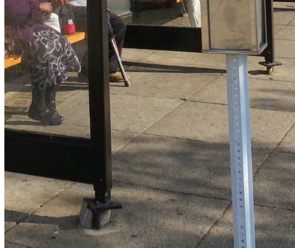
Figure 23: Cracked Pads/Footings, Shelter B
