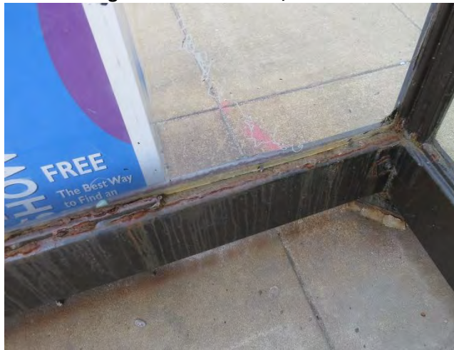
Figure 66: Frame Rust, Shelter F
