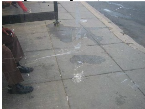
Figure 160: Damaged Panel, Shelter H
