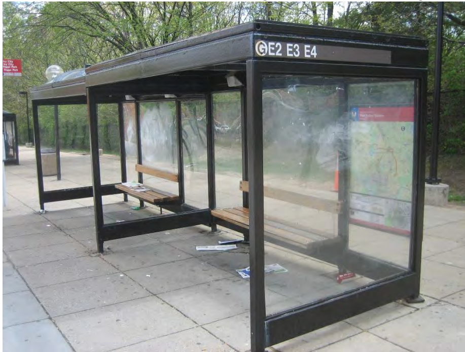
Figure 72: Poor Condition of Shelter G, Missing Panels, Rust and Missing Dome Top
