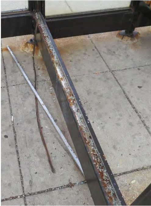
Figure 165: Shelter B West Missing Panel
