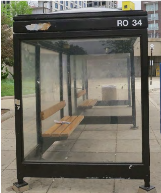
Figure 193: Frame Rust, Shelter F
