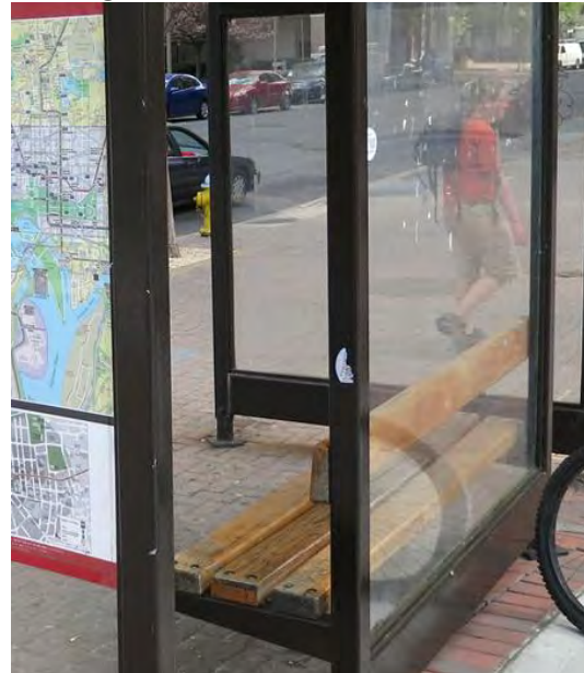
Figure 17: Worn Bench, Shelter H
