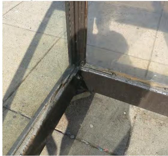
Figure 21: Rusted Frame, Shelter C
