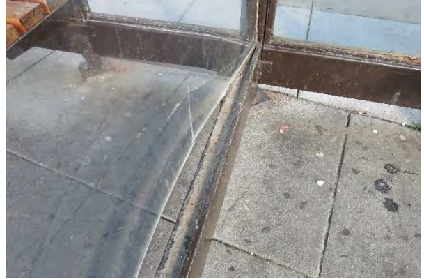
Figure 115: Damaged Panel, Shelter D
