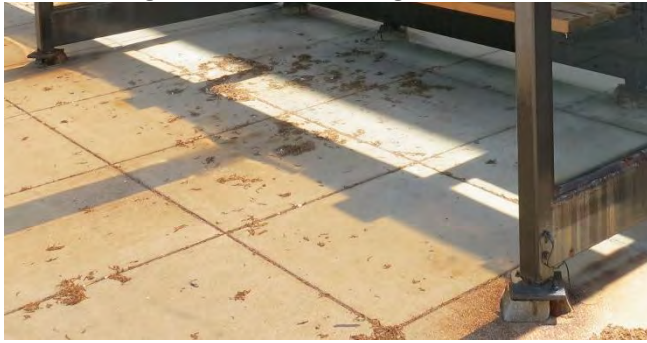
Figure 68: Pad Cracking, Shelter D
