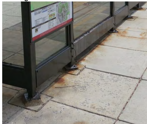
Figure 90: Rust on Frame of Shelter E
