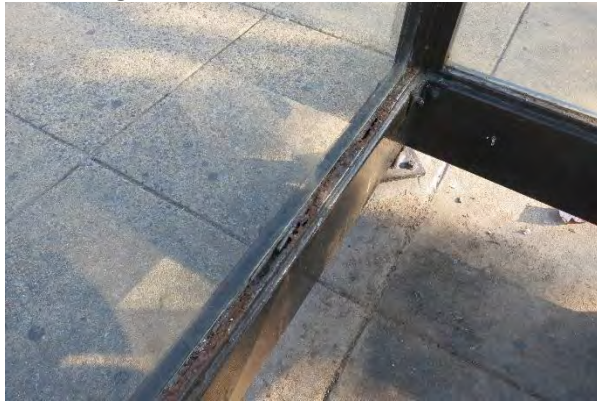
Figure 10: Rusted Frame, Shelter K
