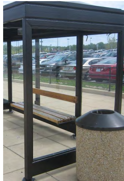
Figure 33: Missing Panel & Worn Bench, Shelter B
