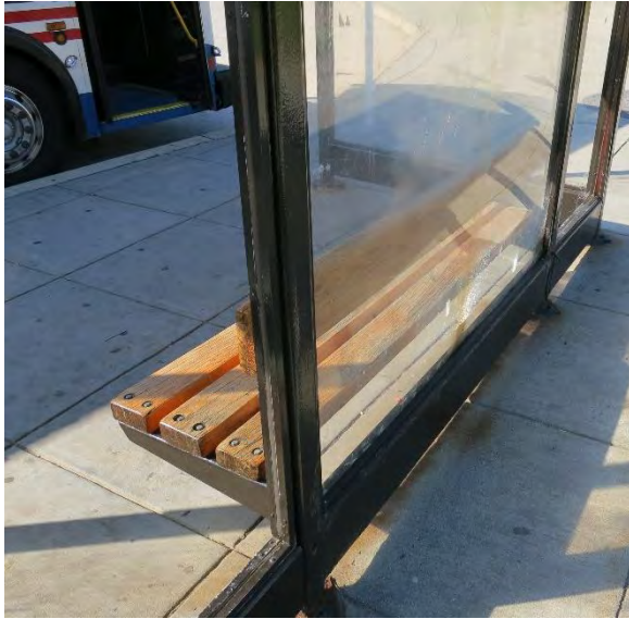
Figure 57: Missing Panel and Frame Rust, Shelter D
