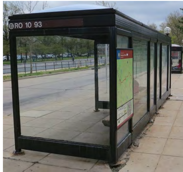
Figure 168: Shelter B East Poor Pad Condition
