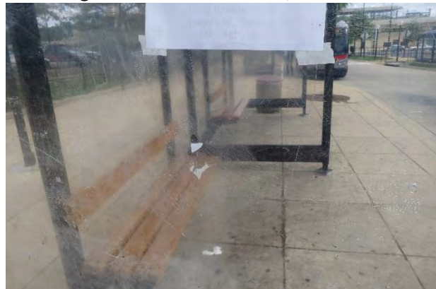
Figure 119: Cracked Panel, Shelter G
