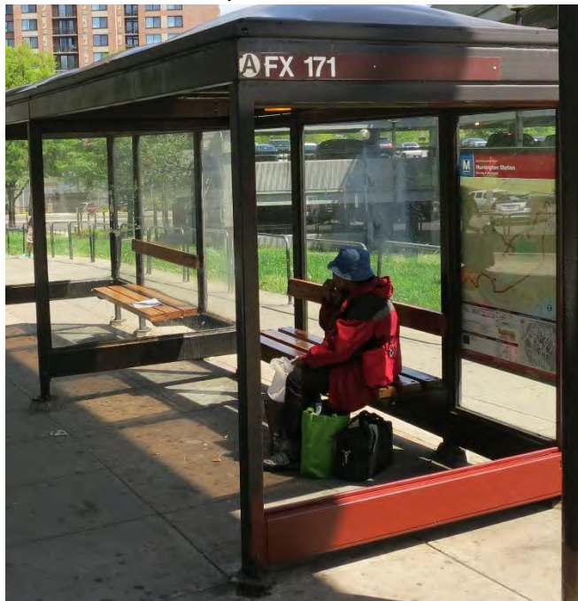
Figure 94: Missing Panel, Cracked Pad and Frame Rust, Shelter A North
