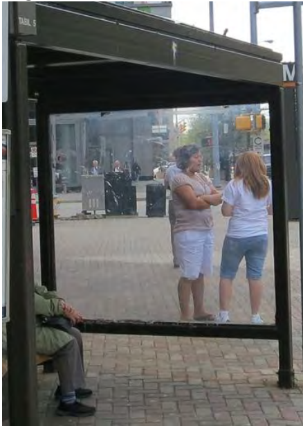
Figure 16: Rusted Frame, Shelter E
