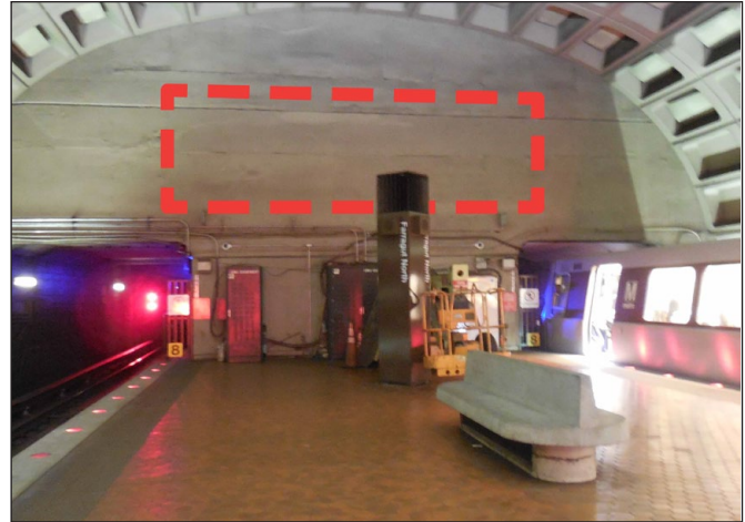
Farragut North Station, southern end of platform, location of pedestrian tunnel connection
