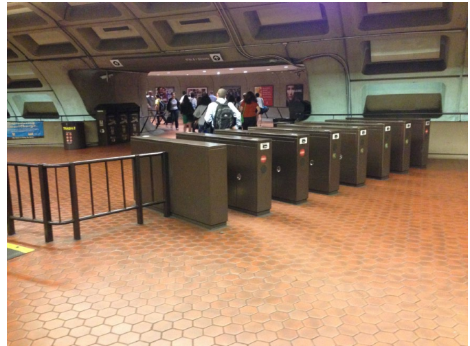
East Mezzanine Faregates (array on south side of kiosk), looking towards the East Entrance passageway
