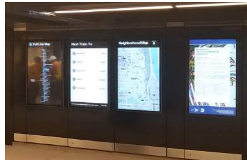
NYC MTA 163 Street Subway Station mezzanine dashboards. Customized product design with 55" standard LCD screen. Subway Route Map, schedule, neighborhood bus map, and service alerts are all integrated into the digital dashboard wall at mezzanine to reduce visual clutter.
