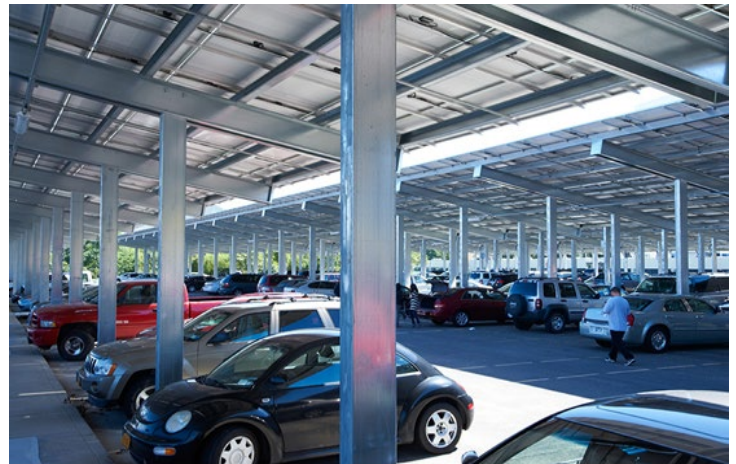
Example of Solar Parking Canopies
