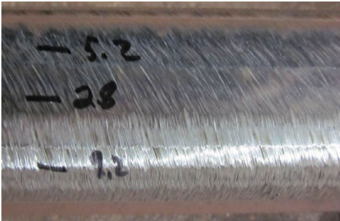
Figure 32 Photograph of right ground rail (guage corner at bottom) ( [REDACTED] "WMATA Post-Grind Surface Roughness Report", Loram Maintenance of Way, December 2013, Figure 2 of Page 2)
