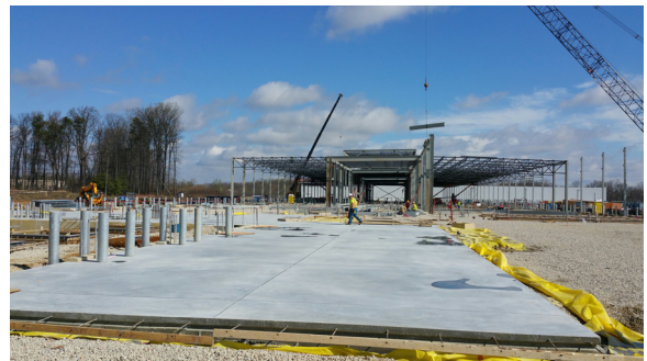
This facility is planned to go into service in FY2020.
