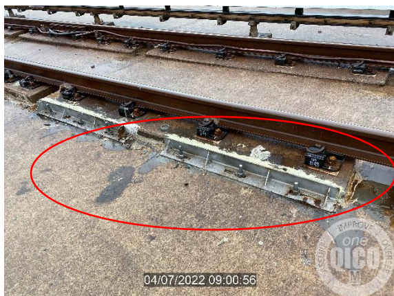
Figure 4: Temporary repairs performed on grout pads located near G1 CM 619+00
