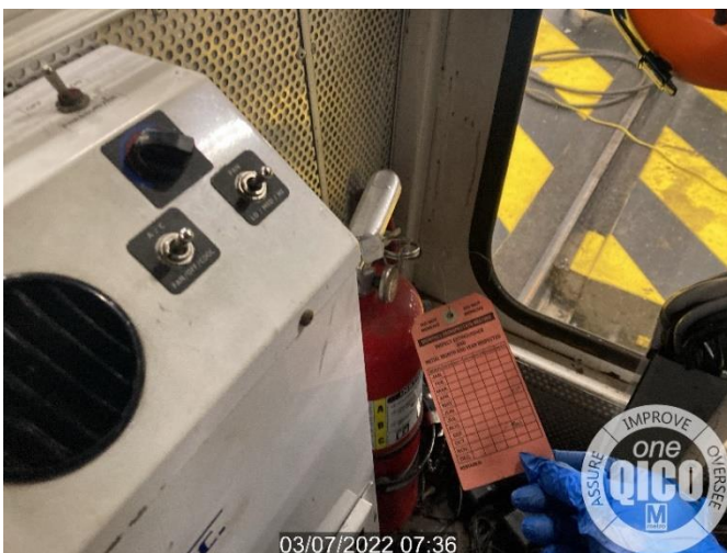
Figure 10: Fire extinguisher inside a Tamper cabin (last inspected June 2019)
