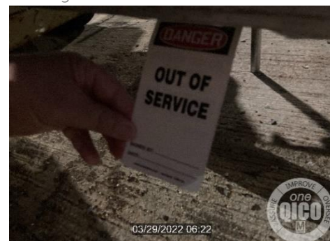
Figure 11: Out of service tag located on rail cart
