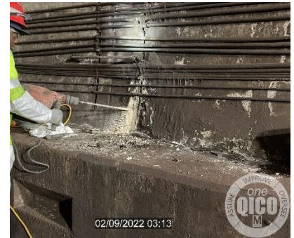
Figure 5: Worker not wearing a mask while drilling into the concrete
