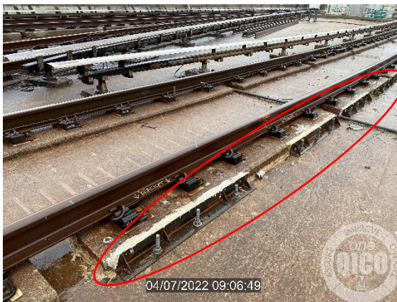
Figure 5: Temporary repairs performed on grout pads
