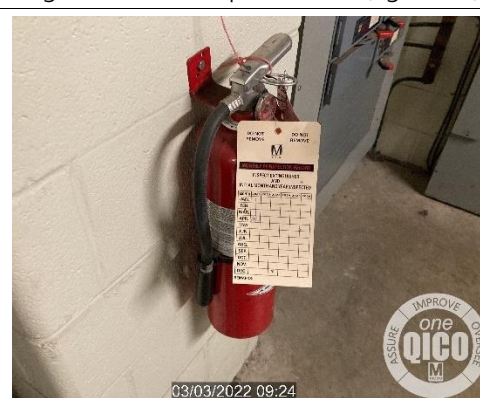
Figure 07: Fire extinguisher last inspected Apr. 2021
