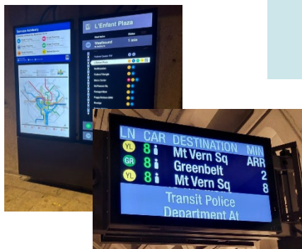
MetroPulse and Passenger Information Display System
