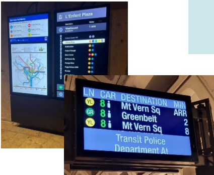
MetroPulse and Passenger Information Display System
