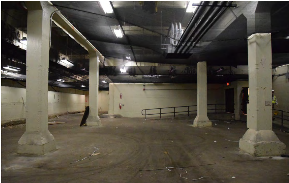
Figure 16. Lower level of the bus garage; the original columns and ceiling are present, however, the concrete floor was removed and excavated in the 1980s. The new concrete footings below the columns are visible in the photo (BBB)
