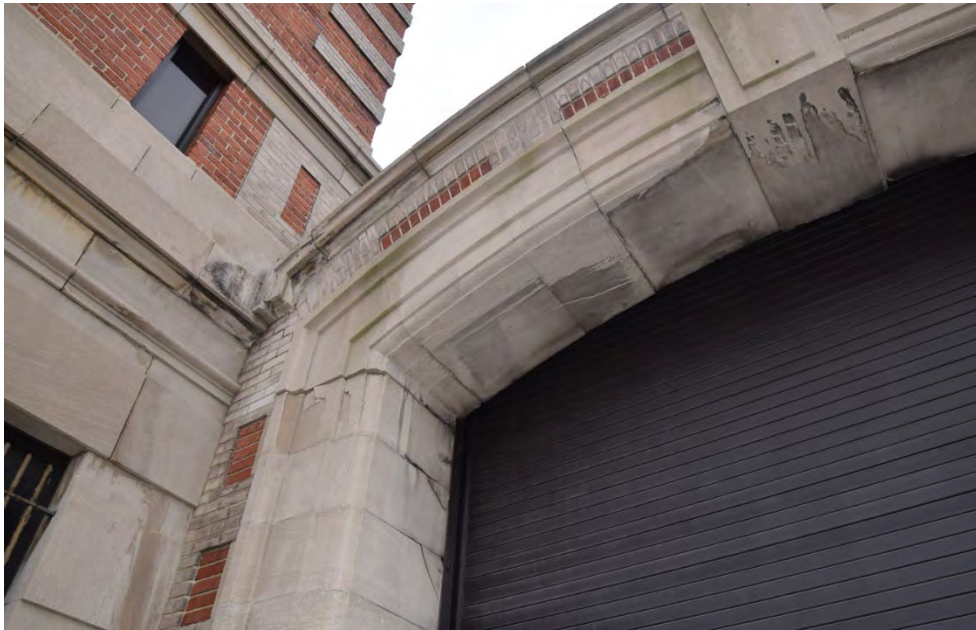
Figure 17. The north facing streetcar/bus opening adjacent to the tower exhibits stone cracking, spalling, and masonry soiling which require repair (BBB)
