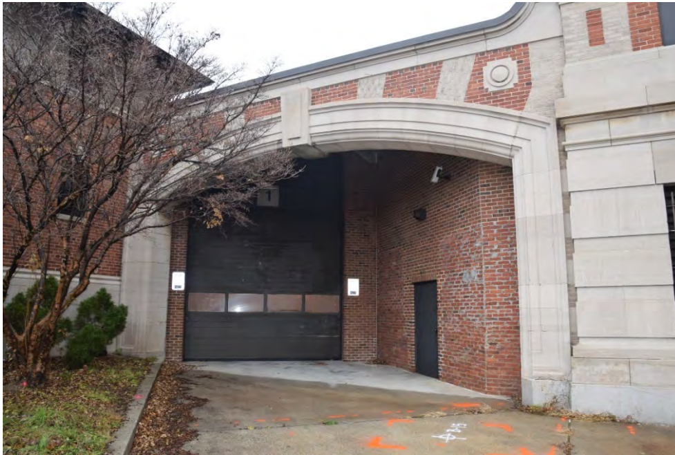
Figure 8. Angled brick wall on right constructed sometime after 1914 and prior to 1978. The other angled wall with the overhanging door was added after 1978 (BBB)
