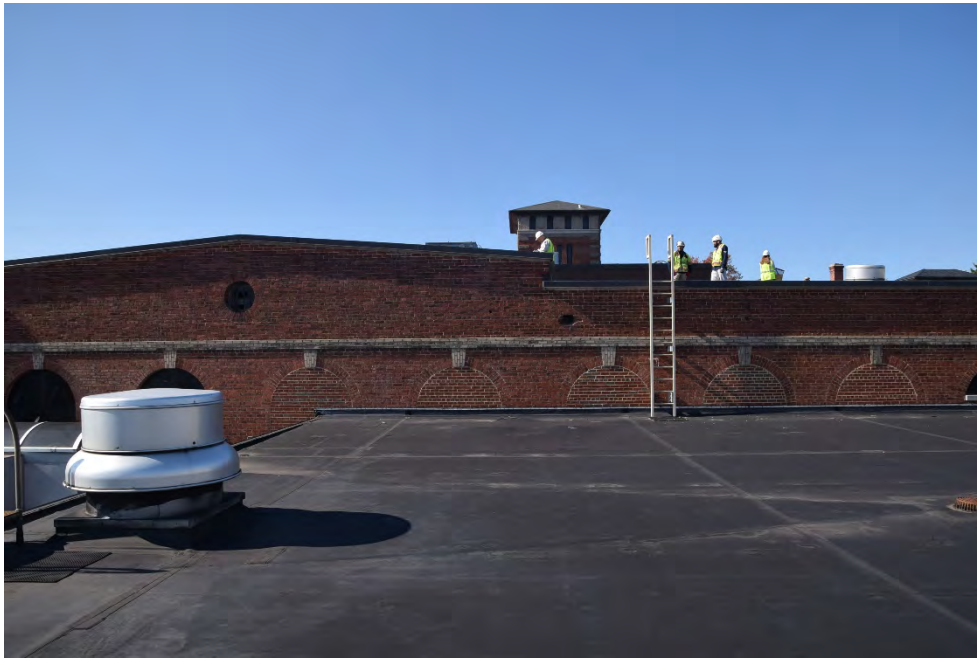
Figure 15. Roof of the 1987 addition abuts the original east elevation. Several of the arched windows have been infilled with brick (BBB)
