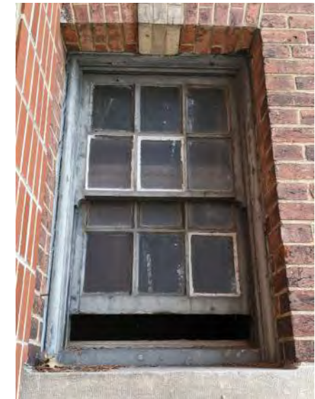
All sash, frame, and muntin profiles to match the only remaining original window on site.
