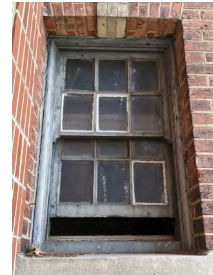
All sash, frame, and muntin profiles to match the only remaining original window on site.
