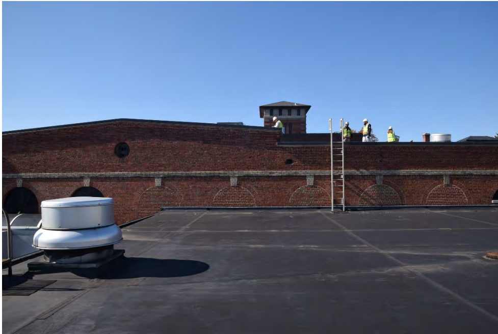
Figure 15. 1987 roof addition abuts original east elevation. Several arched windows infilled with brick (BBB)
