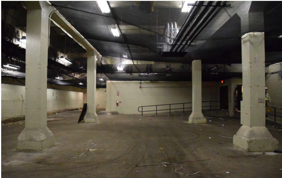
Figure 16. Lower level of the bus garage; the original columns and ceiling are present, however, the concrete floor was removed and excavated in the 1980s. The new concrete footings below the columns are visible in the photo (BBB)
