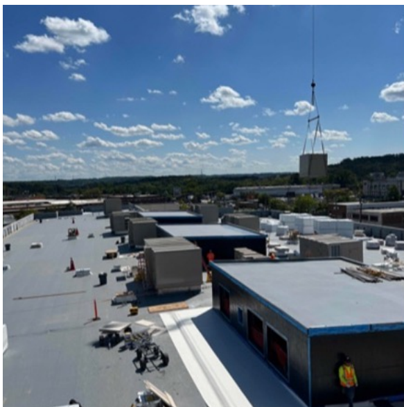
All mechanical roof top equipment set
