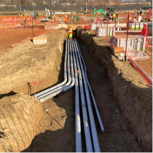
Continuation of Underground Ductbank
