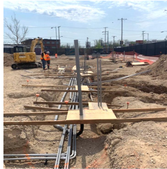
CNG Equipment Feeds
