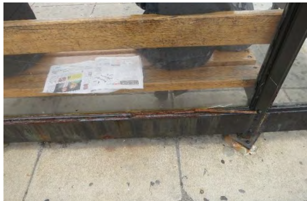
Figure 140: Shelter C East Poor Pad Condition
