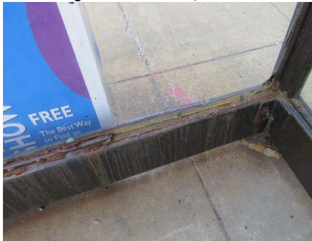
Figure 66: Frame Rust, Shelter F
