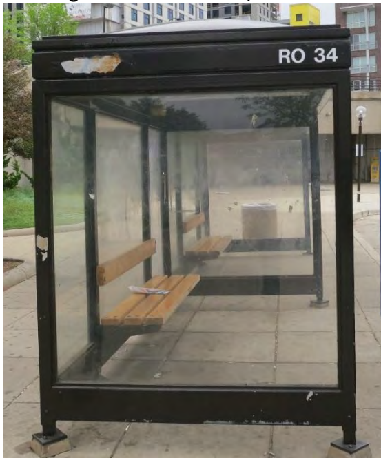
Figure 193: Frame Rust, Shelter F
