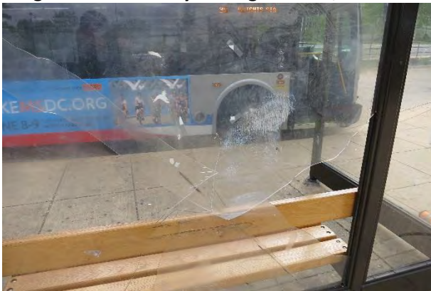
Figure 118: Severely Damaged Panel, Shelter F
