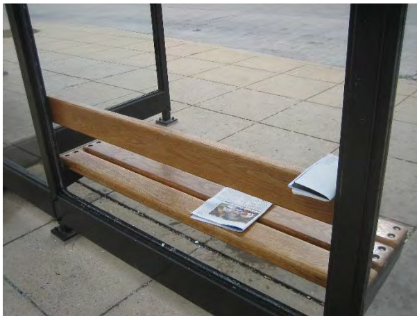
Figure 84: Missing Panel, Shelter B
