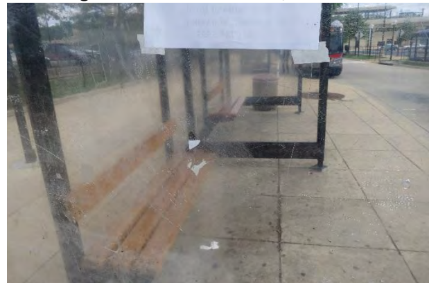
Figure 119: Cracked Panel, Shelter G
