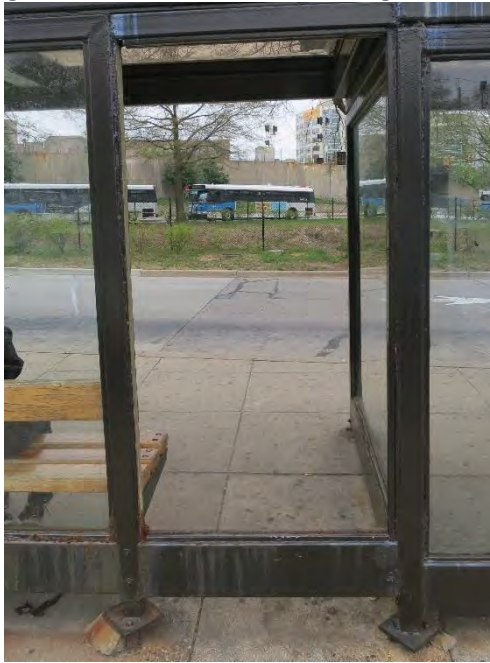
Figure 137: Shelter C East Missing Panel
