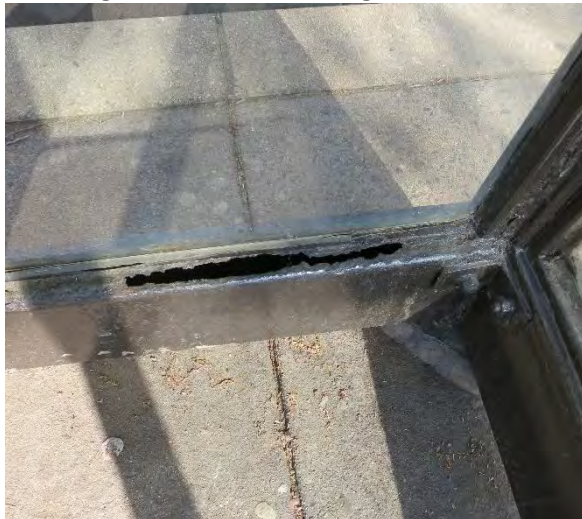
Figure 20: Frame Damage, Shelter B
