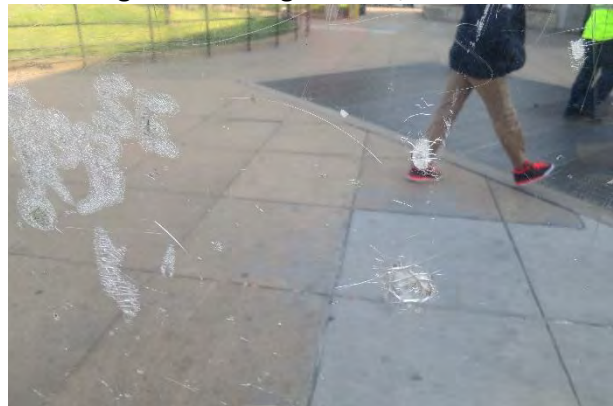
Figure 9: Damaged Panel, Shelter H
