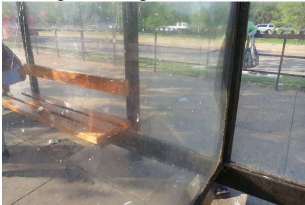
Figure 8: Damaged Panel, Shelter B
