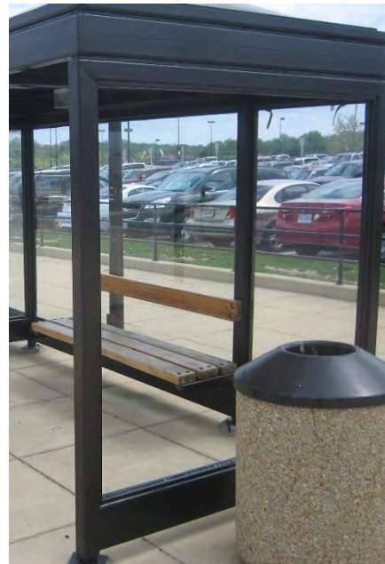
Figure 33: Missing Panel & Worn Bench, Shelter B
