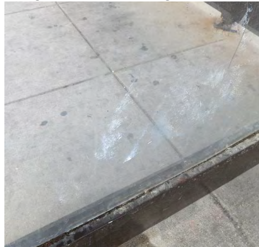
Figure 126: Panel Damage, Shelter A
