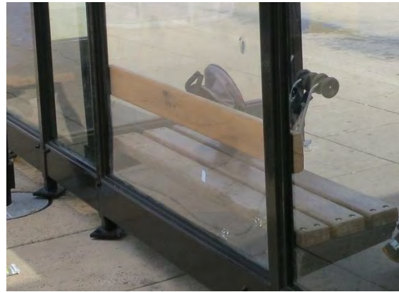
Figure 156: Worn Bench, Cracked Panel, Shelter L
