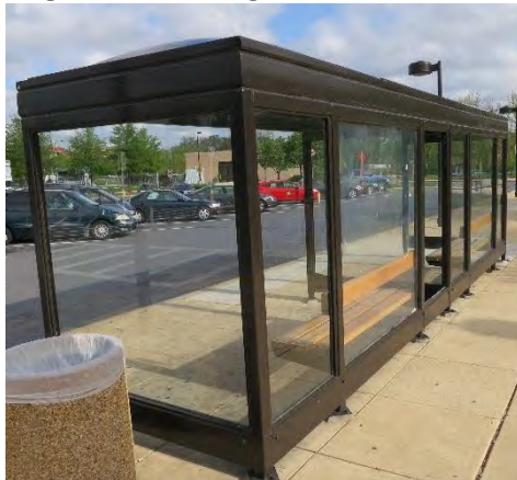
Figure 51: Missing Panel, Kiss & Ride
