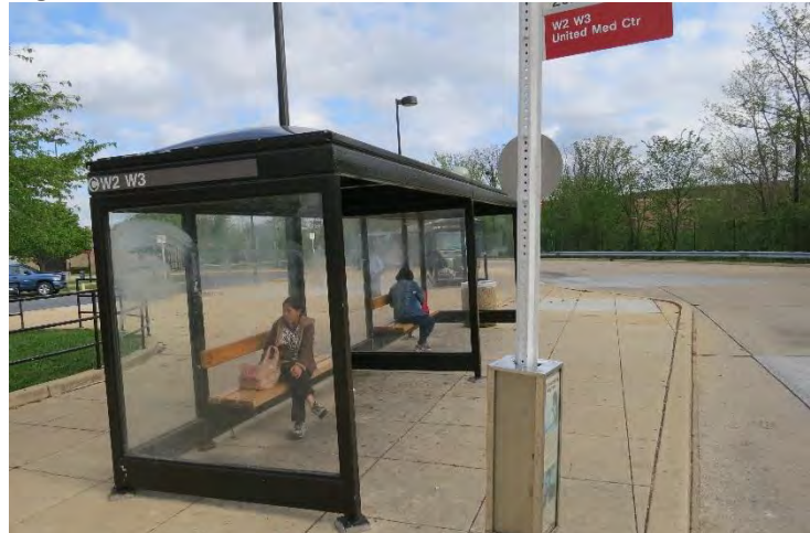
Figure 52: Smeared Panel, Good Frame Condition, Shelter C
