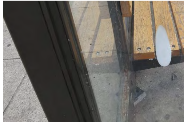
Figure 151: Frame Rust, Damaged Panel, Shelter M
