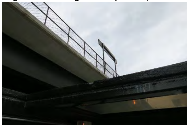
Figure 131: Missing Dome Top & Rust, Shelter C
