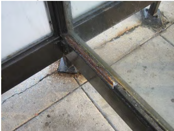
Figure 159: Frame Rust, Shelter B
