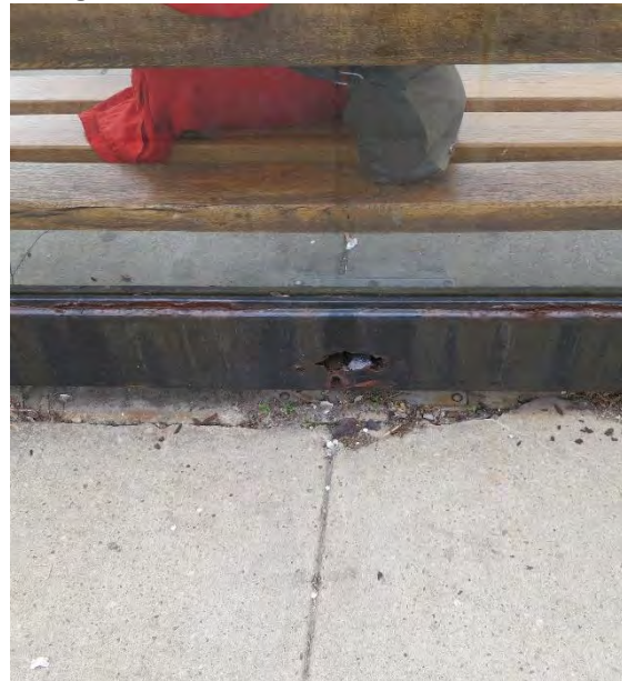
Figure 144: Shelter C East Hole in Frame
