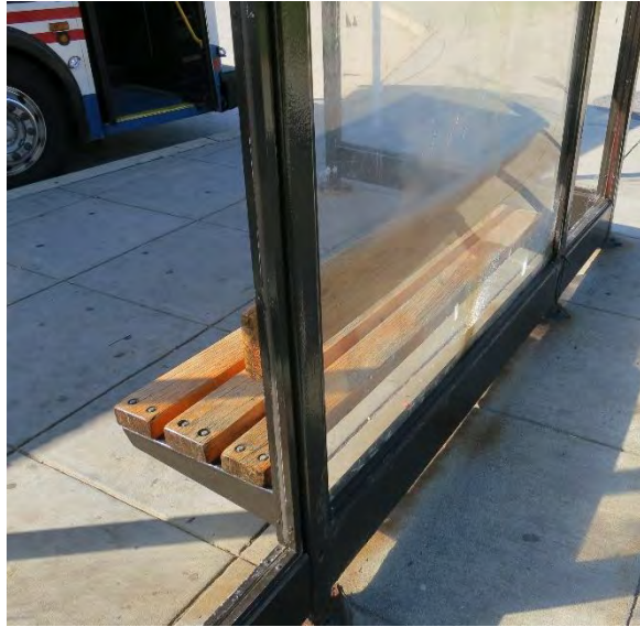
Figure 57: Missing Panel and Frame Rust, Shelter D
