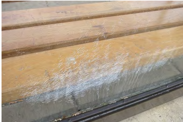
Figure 150: Damaged Panel, Shelter C
