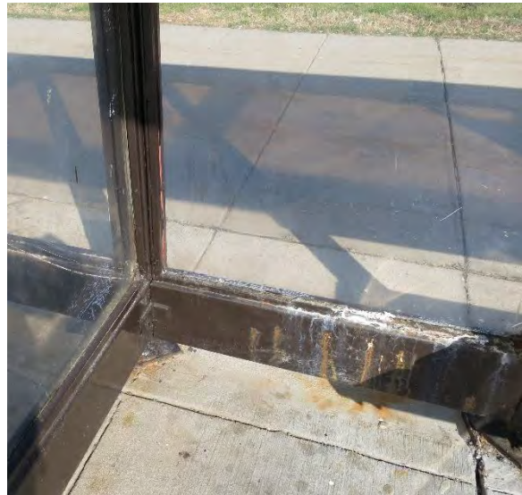
Figure 56: Frame Rust, Shelter C
