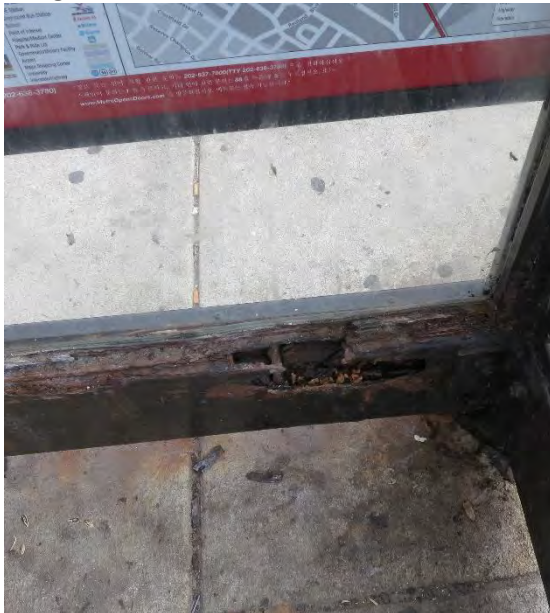
Figure 143: Shelter C West Hole in Frame
