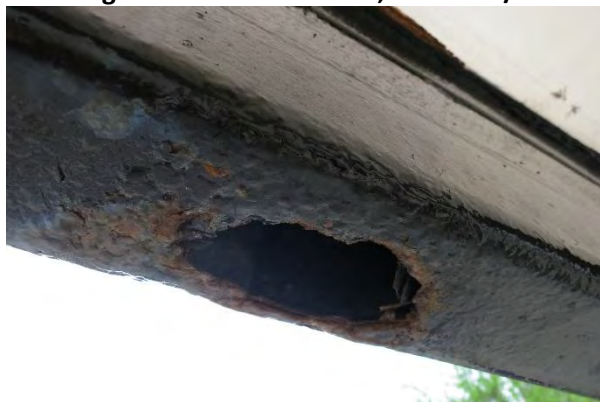
Figure 27: Hole in Frame, Shelter D/J
