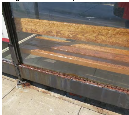
Figure 97: Frame Rust, Shelter D North
