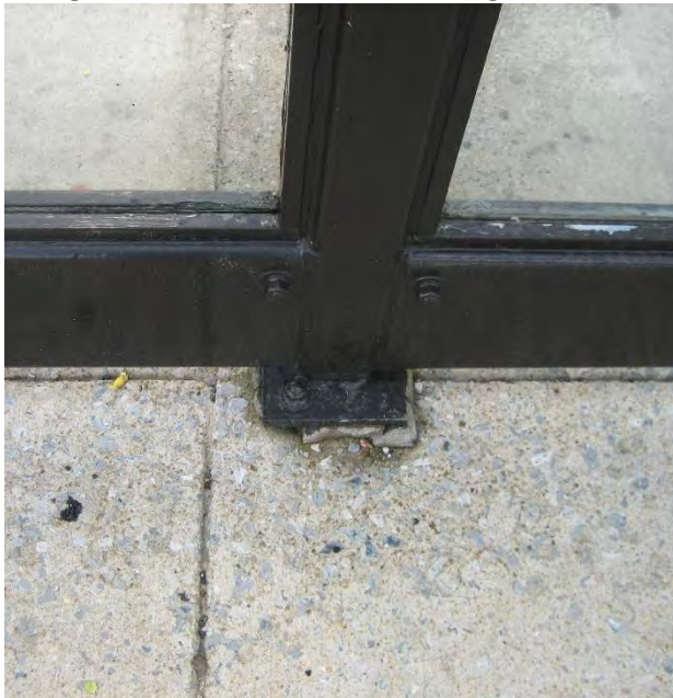
Figure 184: Cracked Pad & Footing, Shelter C
