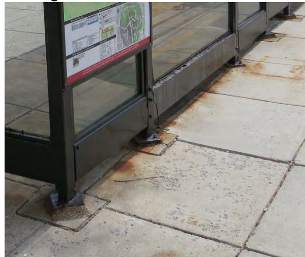
Figure 90: Rust on Frame of Shelter E
