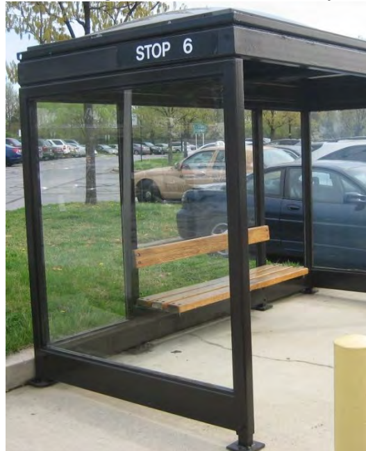
Figure 86: Missing Panel, Park-and-Ride Stop 6 Shelter
