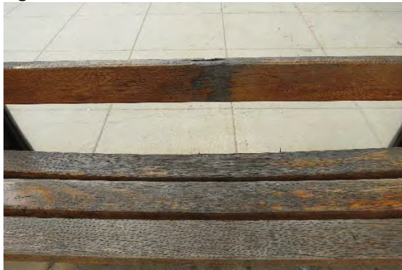
Figure 167: Shelter F East Poor Bench Condition
