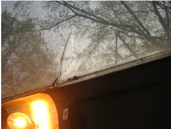
Figure 161: Cracked Dome Top, Shelter G
