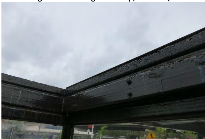
Figure 29: Missing Dome Top, Shelter E/H
