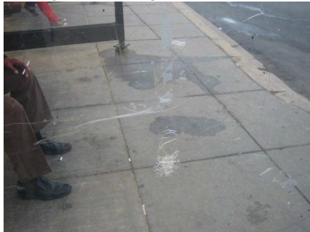
Figure 160: Damaged Panel, Shelter H
