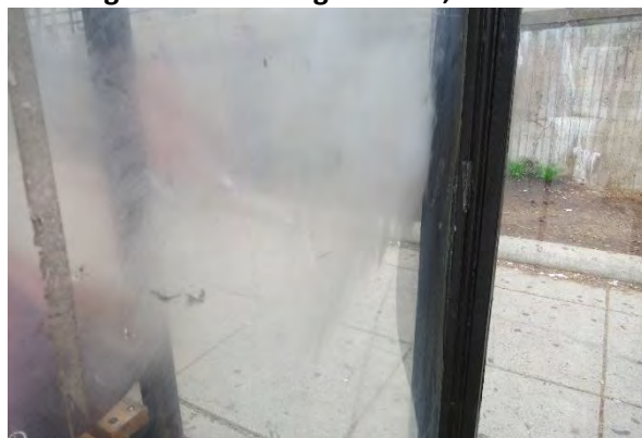
Figure 192: Damaged Panel, Shelter D
