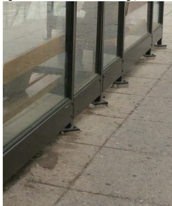
Figure 194: Cracked Pad & Footings, Shelter G
