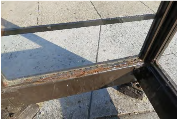
Figure 114: Frame Rust, Shelter B
