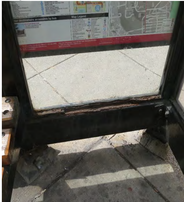
Figure 106: Poor Frame Condition, Shelter D
