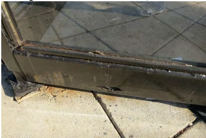
Figure 123: Rust & Hole in Frame, Shelter G
