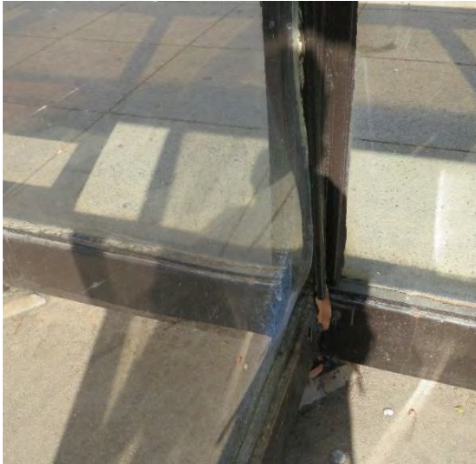
Figure 22: Damaged Panel, Shelter E
