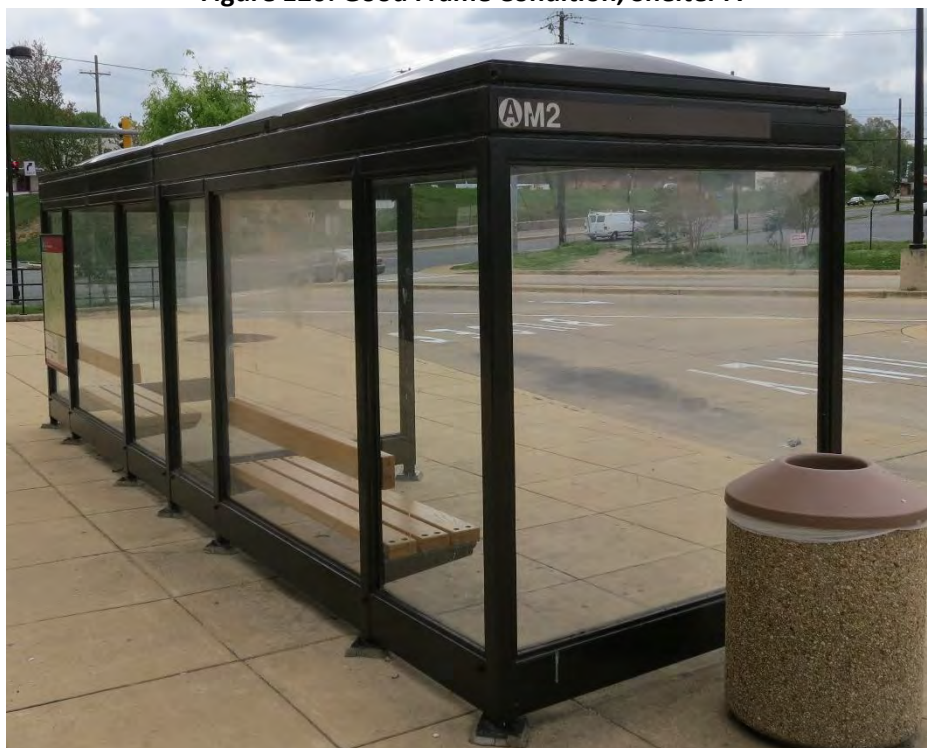
Figure 120: Good Frame Condition, Shelter A
