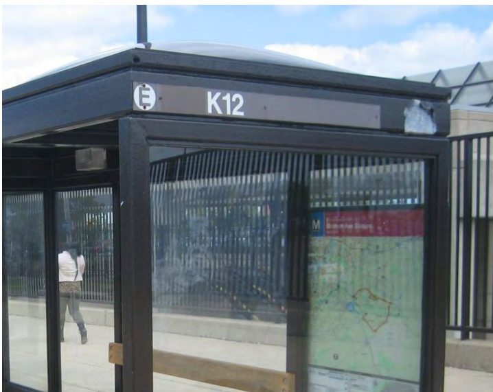
Figure 34: Peeling Paint, Shelter E
