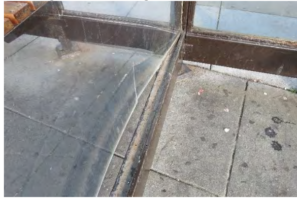
Figure 115: Damaged Panel, Shelter D
