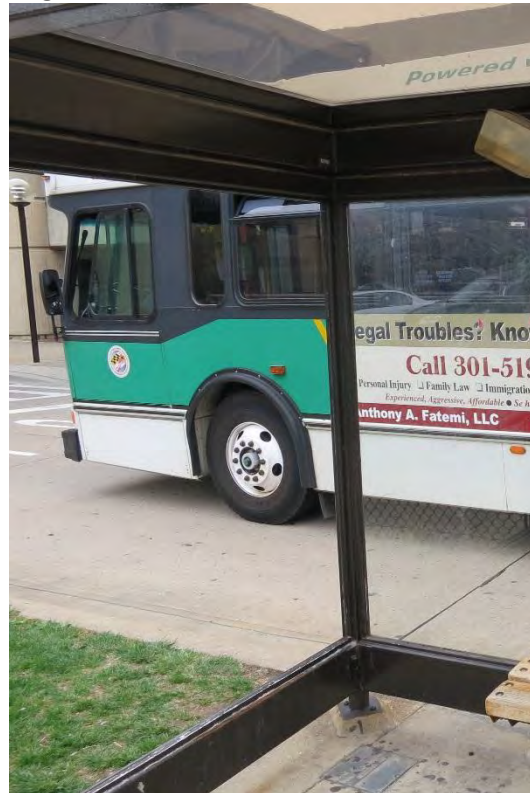
Figure 138: Shelter B West Rust on Frame
