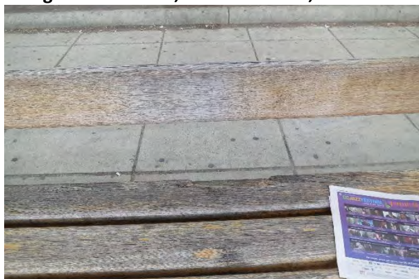
Figure 191: Worn, Cracked Bench, Shelter B
