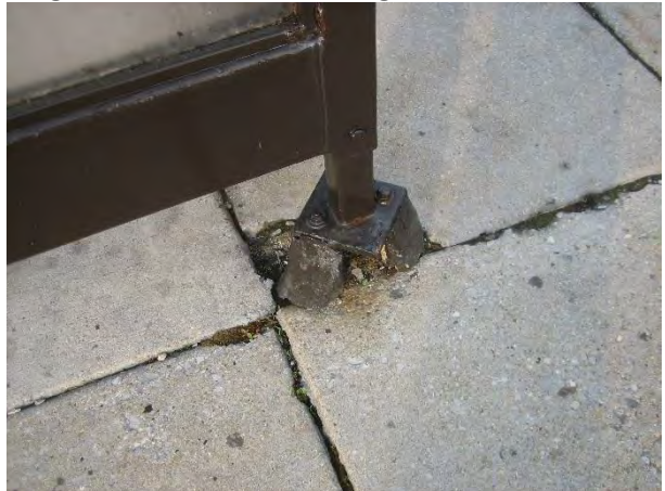
Figure 162: Cracked Footing and Pad, Shelter B
