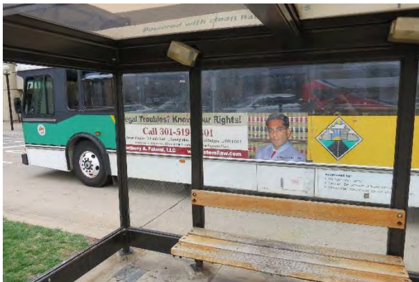
Figure 139: Kiss-and-Ride Shelter Missing Panel
