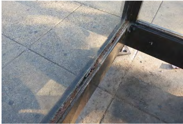
Figure 10: Rusted Frame, Shelter K
