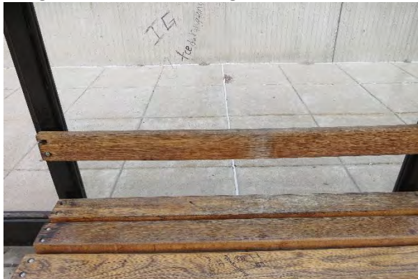
Figure 148: Worn/Damaged Bench, Shelter K
