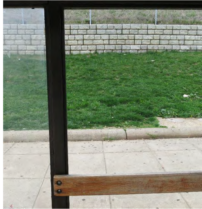
Figure 166: Shelter A East Missing Panel
