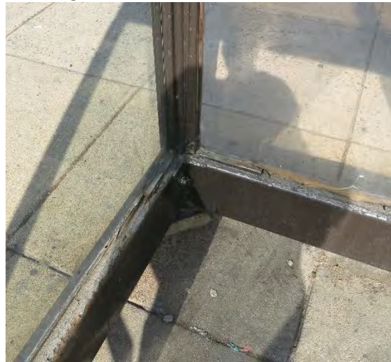
Figure 21: Rusty Frame, Shelter C
