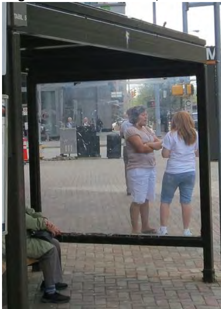
Figure 16: Rusty Frame, Shelter E
