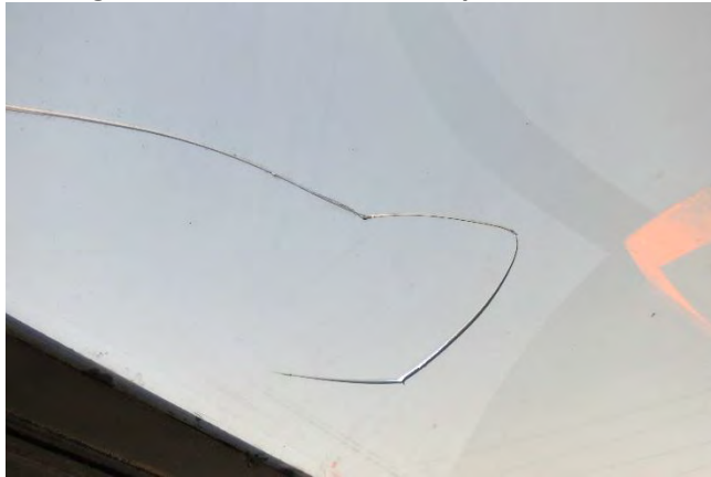
Figure 125: Cracked Dome Top, Taxi Shelter
