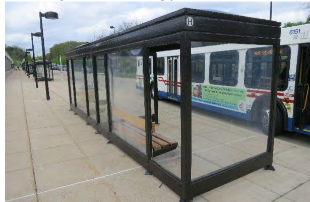
Figure 149: Missing panel, Shelter H
