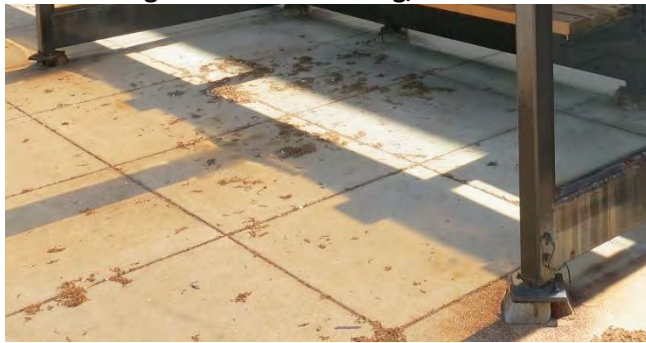
Figure 68: Pad Cracking, Shelter D
