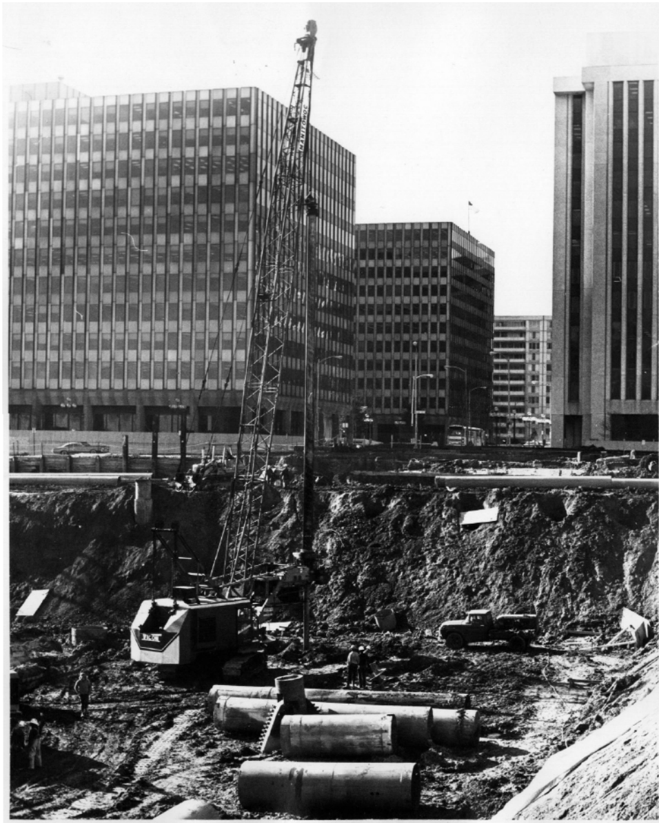
Figure 7: Construction of the Crystal City Metrorail Station circa 1977, looking south across 18th Street (source: Arlington County CPHD)
