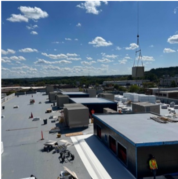
All mechanical roof top equipment set
