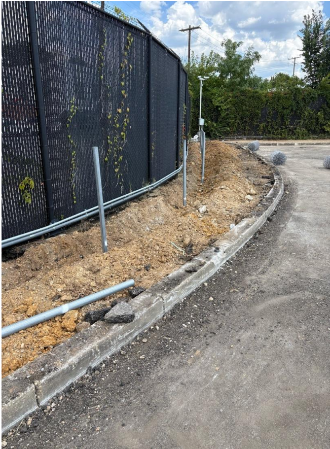
Perimeter Super Silt Fence
