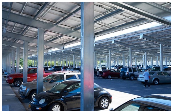
Example of Solar Parking Canopies
