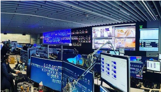
Metro Integrated Command & Communications Center (MICC)
