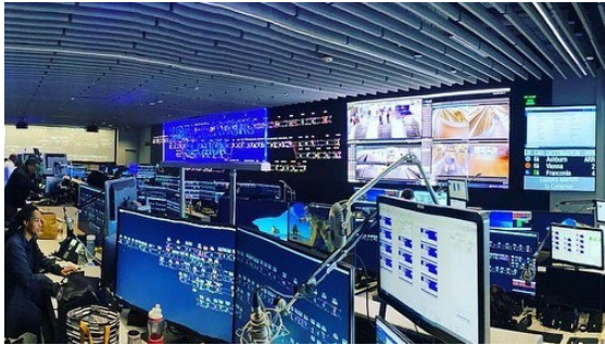
Metro Integrated Command & Communications Center (MICC)
