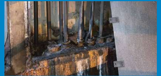
Traction Power Cables
