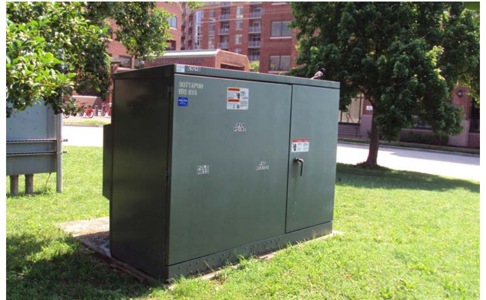
Photo 04 - Non-PCB Pad-Mounted Transformer at Braddock Road Metro Station
