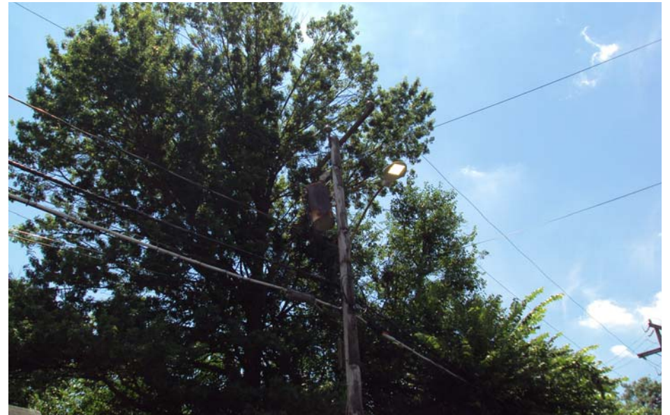
Photo 16 - Pole-Mounted Transformer - N. West Street
