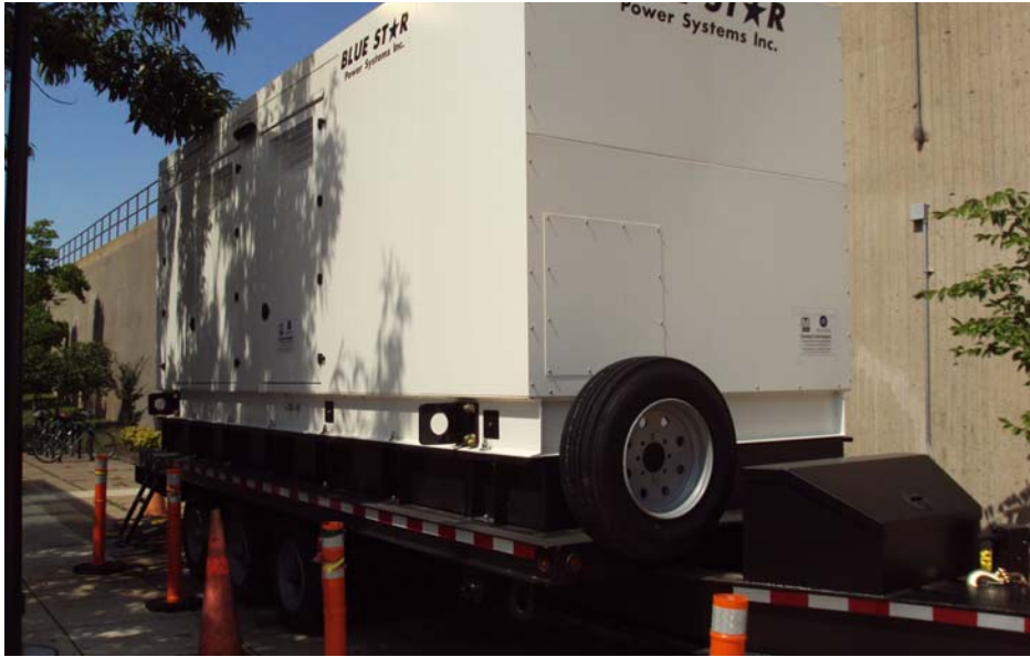
Photo 05 - Portable Generator at Braddock Road Metro Station
