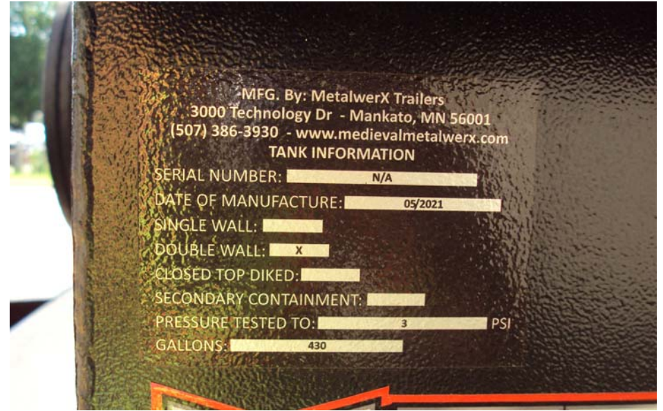
Photo 06 - Portable Generator Placard
