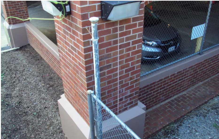
Photo 07 - Vent Pipe at 1320 Braddock Place
