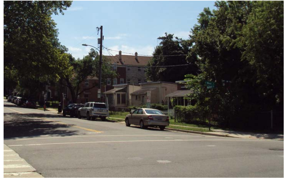
Photo 14 - Pole-Mounted Transformer - Madison Street and N West Street
