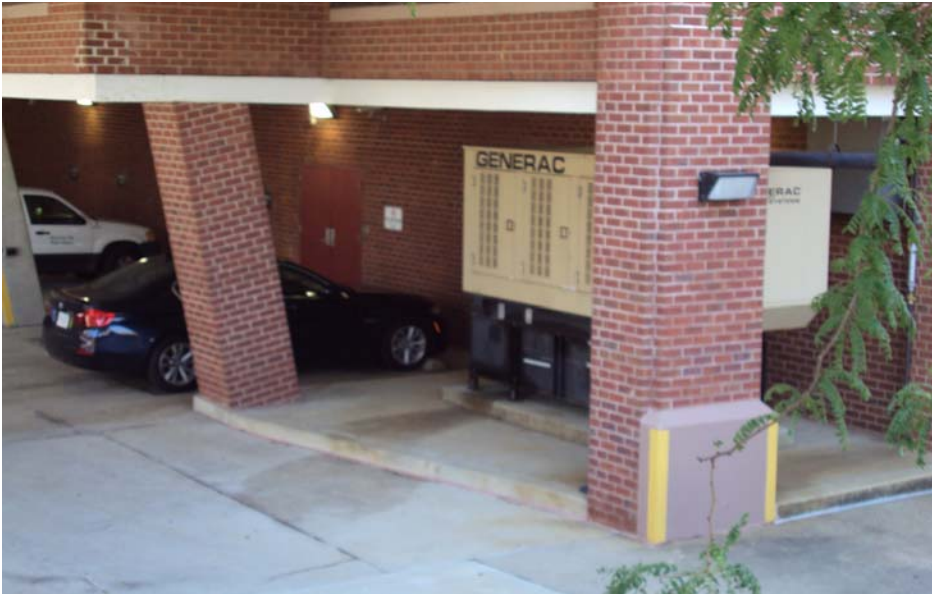
Photo 13 - Emergency Generator with Staining at 1340 Braddock Place
