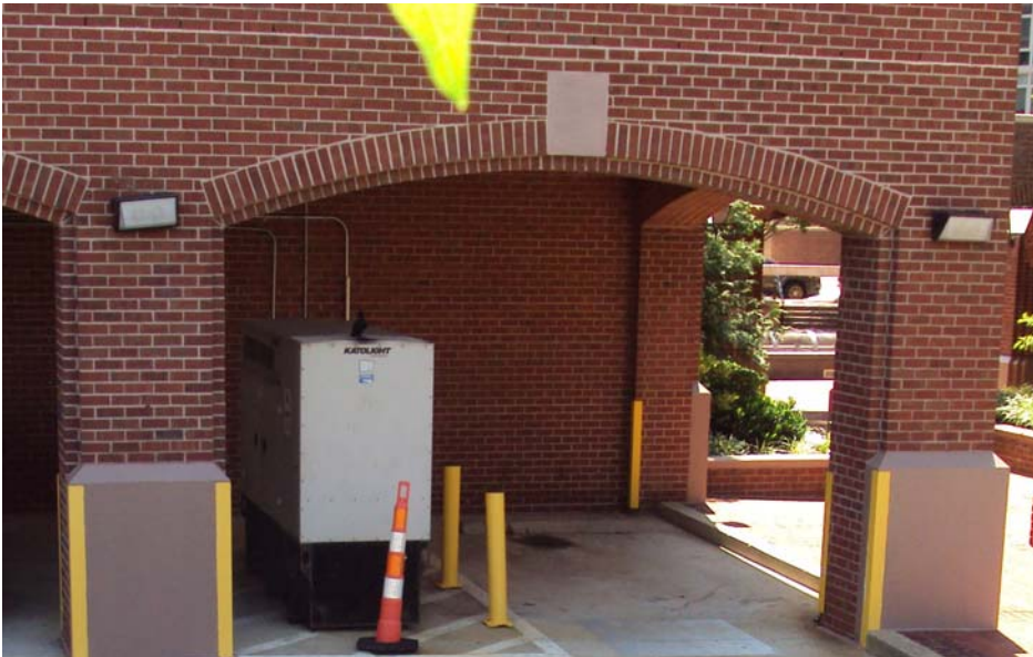
Photo 11 - Emergency Generator No. 1 at 1330 Braddock Place
