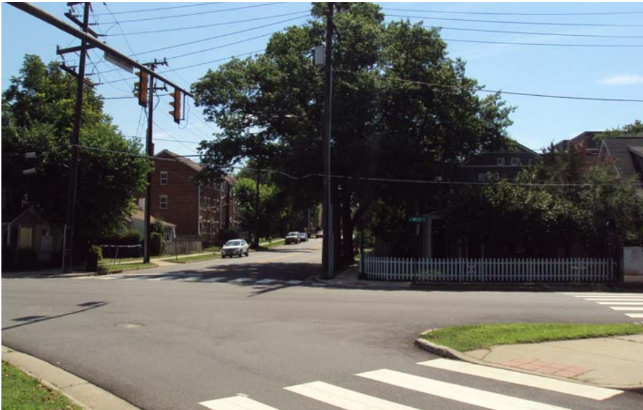
Photo 15 - Pole-Mounted Transformer - N. West and Wythe Street
