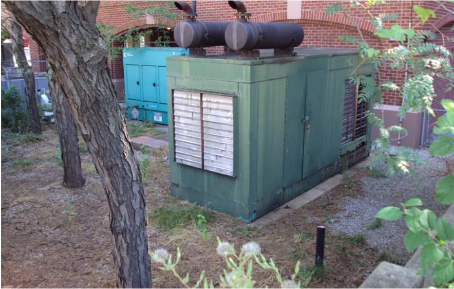
Photo 09 - Emergency Generators at 1320 Braddock Place
