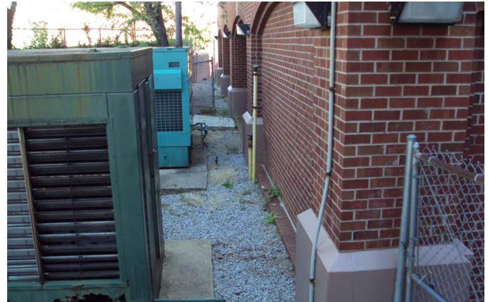
Photo 08 - Vent Pipe and Fill Port at 1320 Braddock Place
