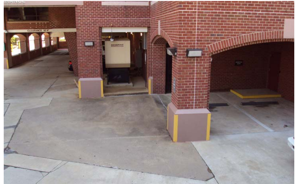
Photo 12 - Emergency Generator No. 2 at 1330 Braddock Place
