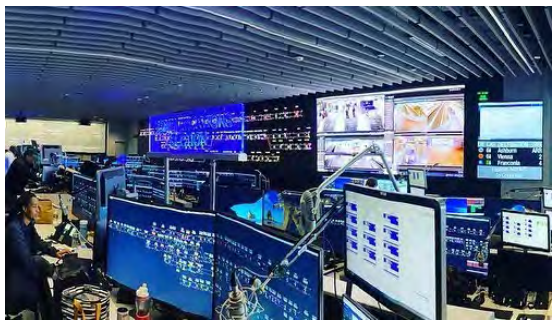
WMATA's Metro Integrated Command and Communications Center (MICC)
