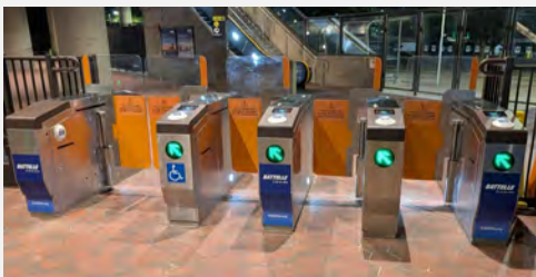
Metro Rail Faregates
