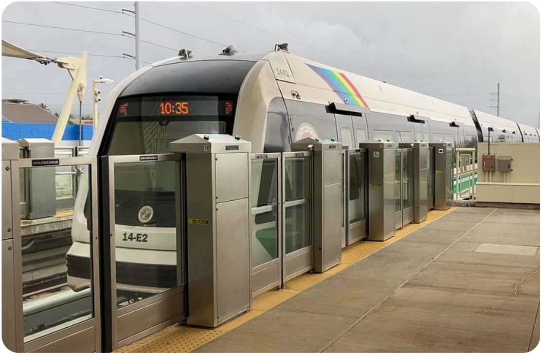
Partial Height Doors - Honolulu Area Rapid Transit (HART)
