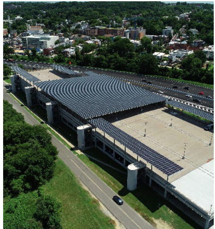
Solar Carports at Anacostia Station Garage (Aug 2022)
