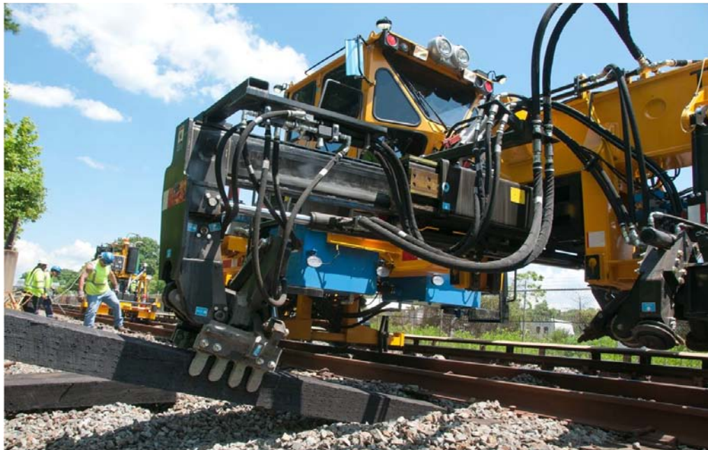
Photo of Track maintenance crew replacing ties on track number 1 between Rockville and Shady Grove using the recently delivered Tie Inserter
