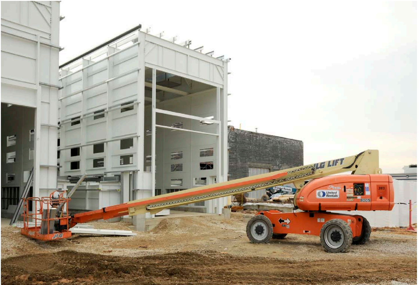
Photo of the new Metro Bus Paint and Body Shop at Carmen Turner Facility, under construction, funded through the American Recovery & Reinvestment Act.
