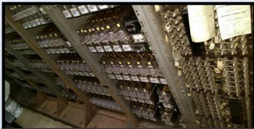
165 Train Control Rooms
