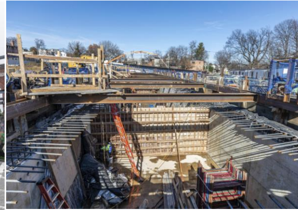
Storm Water Management Tank
