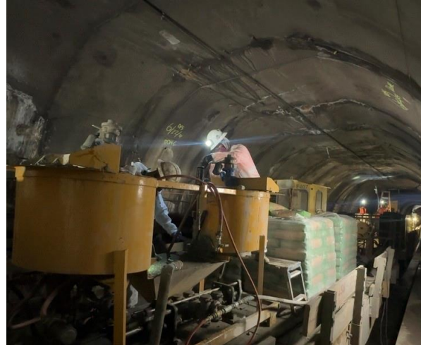
Water Leak Mitigation on Red Line
