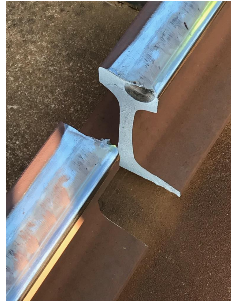
Rail Break and Defect Page 38 of 59
