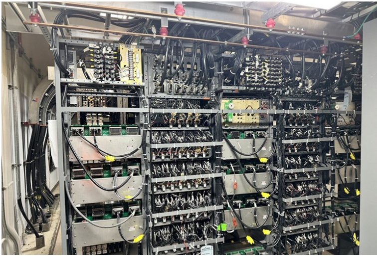
WMATA Red Line Train Control Room
