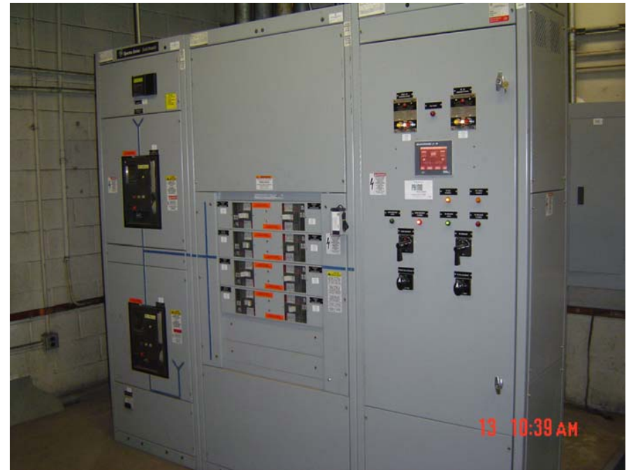
Pentagon City- New AC Switchgear
