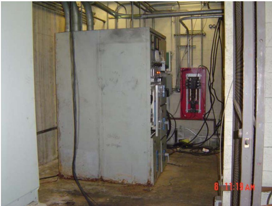
Pentagon City- Old AC Switchgear
