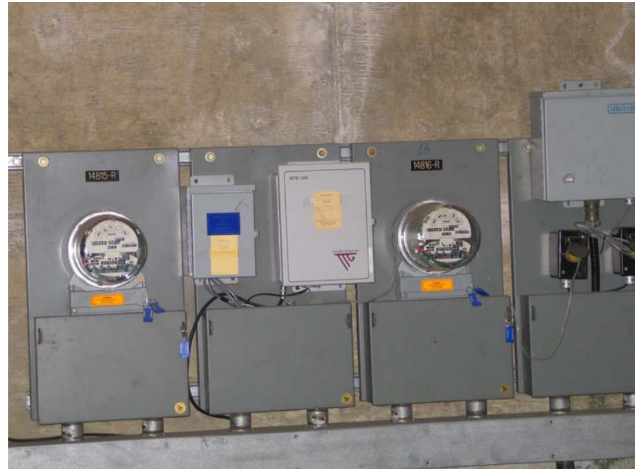
D10- Deanwood new metering system
