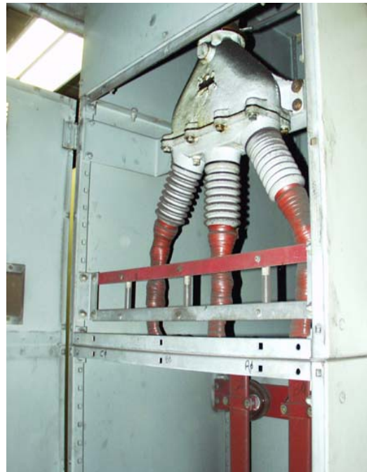
Capitol South - Current lead cable feeds
