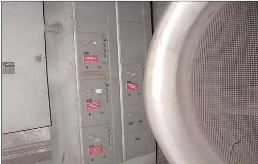
Serves Ventilation Fans & Drainage Pumps
