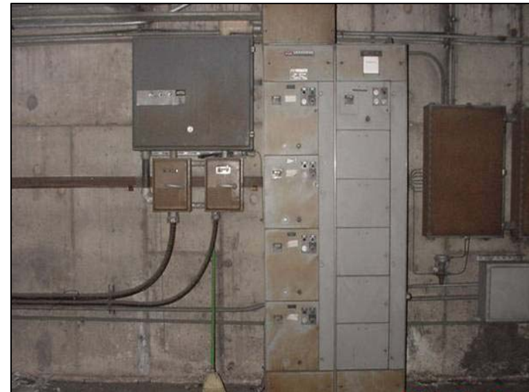
Motor Control Center
