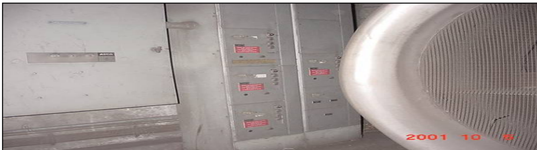
Serves Ventilation Fans & Drainage Pumps
