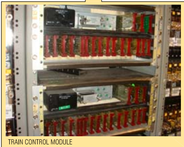
TRAIN CONTROL MODULE
