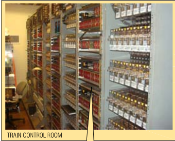
TRAIN CONTROL ROOM
