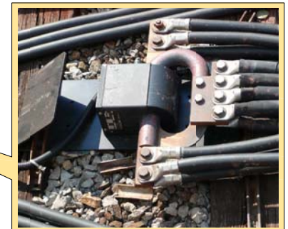
HIGH CURRENT SUBSTATION RETURN IMPEDENCE BOND
