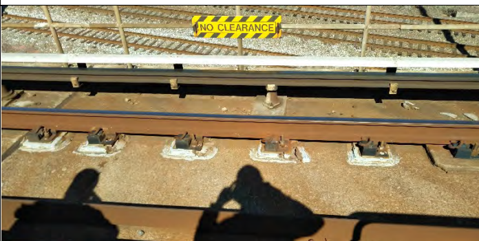
Multiple defective pads and fasteners (BLACK Defect)
