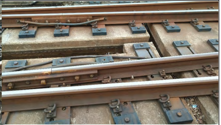
Missing Anchor Bolt
