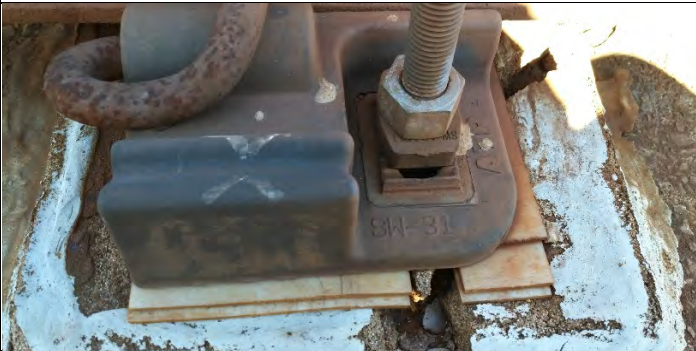
Defective grout pad and fastener
