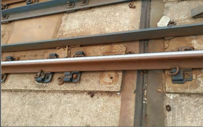
Missing clips and anchor bolts (RED Defect)
