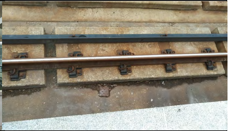
Missing Clip at Largo Platform
