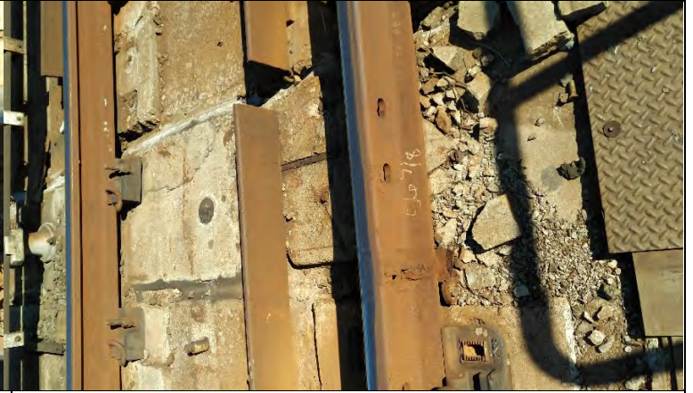
Old deteriorated grout pads and defective EGR
