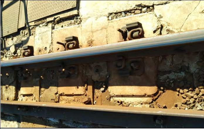
Deteriorated grout pads
