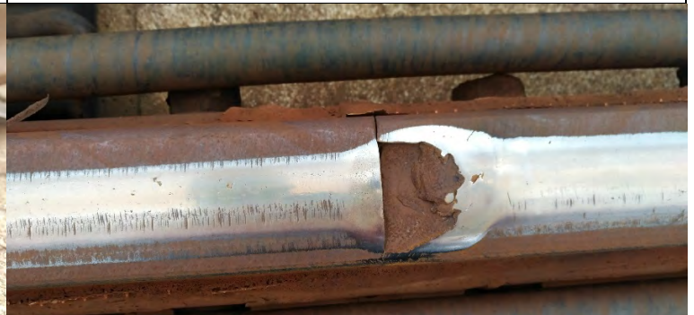
Rail end batter, 0.25" deep, (YELLOW Defect)
