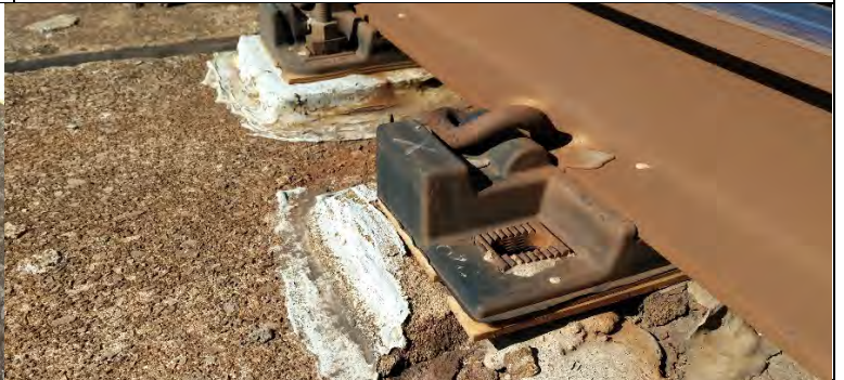
Defective grout pad and fastener
