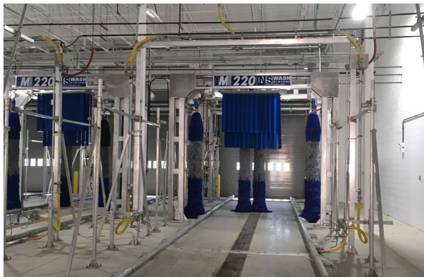
New bus wash bay at Andrews Federal Bus Garage reduces energy and water consumption.
