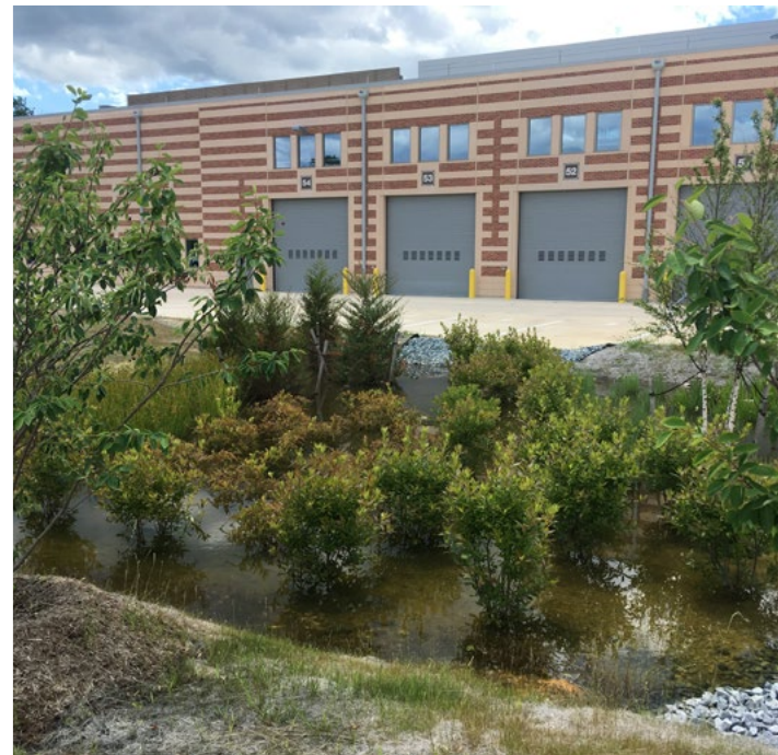
Bottom photo: Rain garden at Andrews Bus Garage
