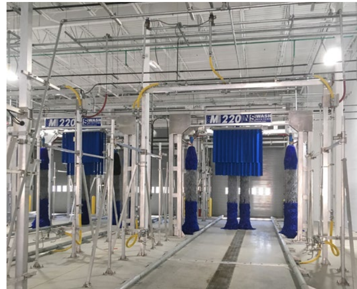
Andrews Bus Garage uses technology that captures, cleans, and reuses stormwater
