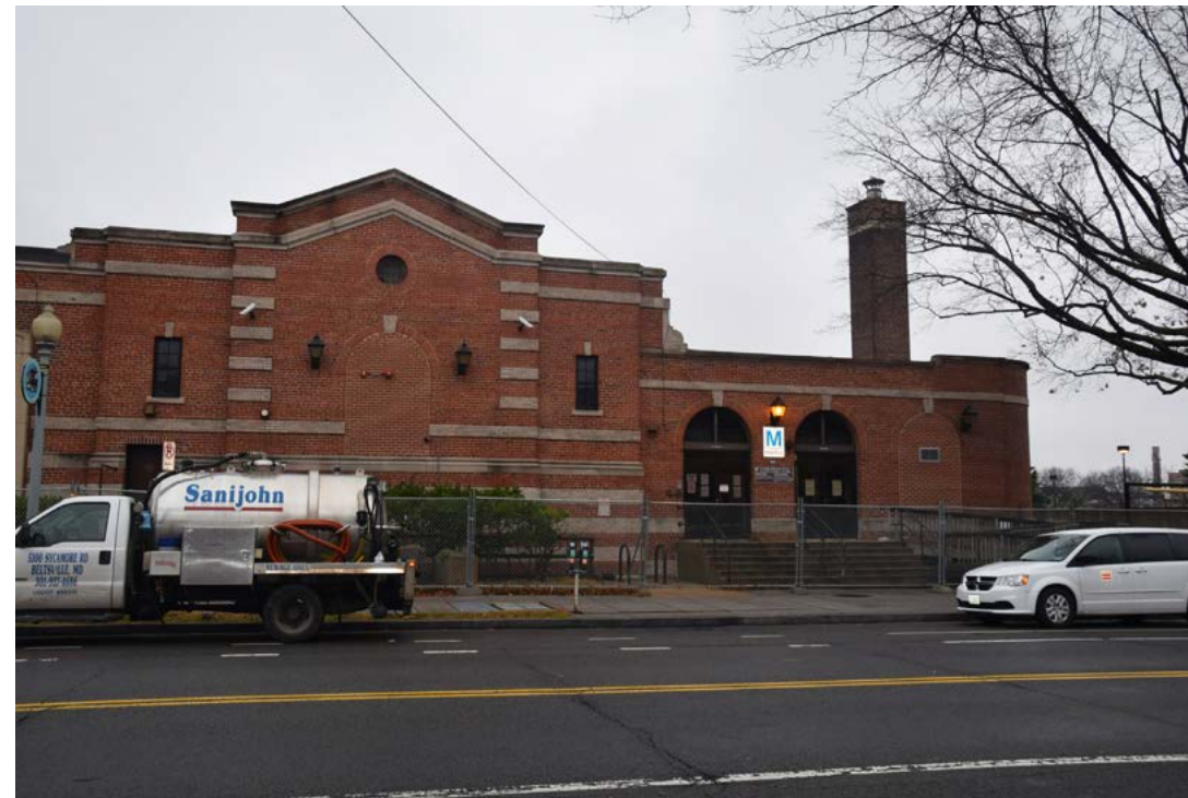
Southern end of west elevation; arched windows have been converted to door and window at center of pedimented bay has been infilled with brick
