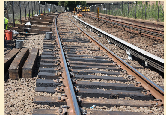
SafeTrack greatly accelerated WMATA's efforts to bring its most deteriorated tracks into a state of good repair. In just six months in 2016, crews replaced over 28,000 crossties, more than 2014 and 2015 combined.
