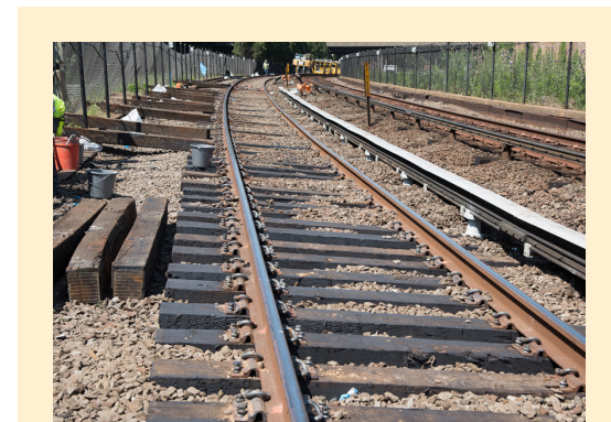
SafeTrack greatly accelerated WMATA's efforts to bring its most deteriorated tracks into a state of good repair. In just six months in 2016, crews replaced over 28,000 crossies, more than 2014 and 2015 combined.
