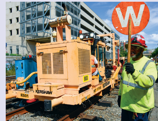
SafeTrack activities require vigilance in safety procedures for the safety of all employees within work zones.
