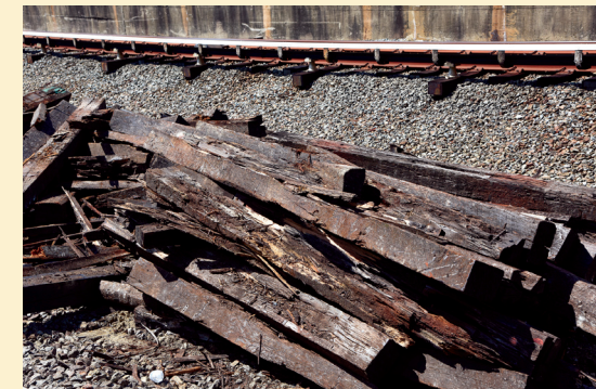
Through Surge 8 (ended September 11, 2016), crews have replaced over 17,000 cross-ties, 10,000 fasteners and 2.4 miles of rail in SafeTrack work areas.
