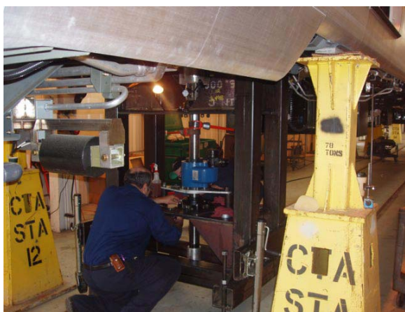
Worker Preparing Boring Machine for Installing New Center Pin at Hornell, NY Facility
