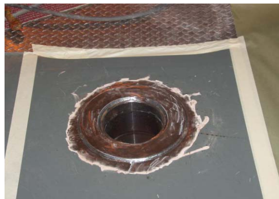
New Center Pin Installed in Railcar Ready for Painting of Railcar Floor
