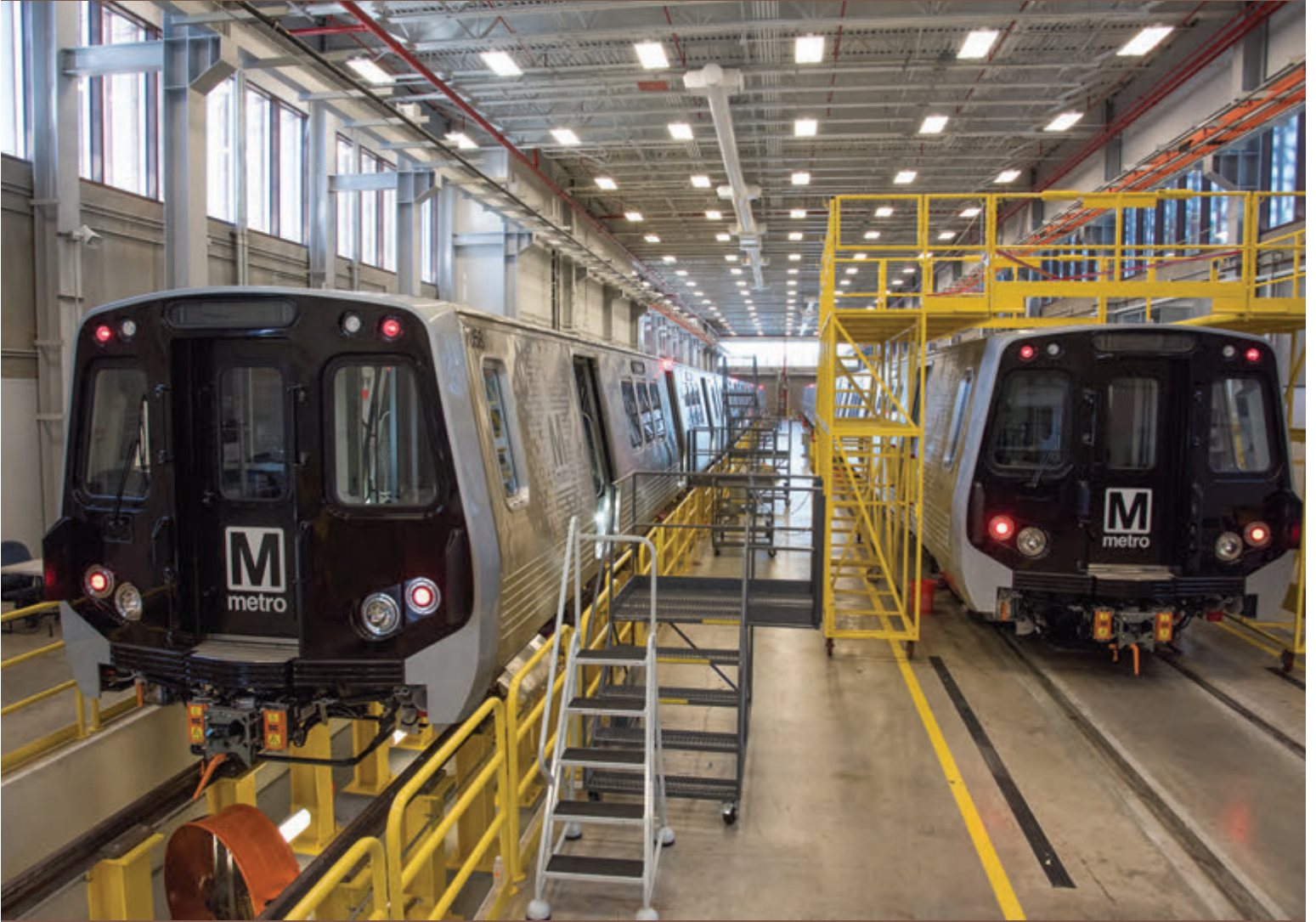
7000 Series Railcar Commissioning Shop
